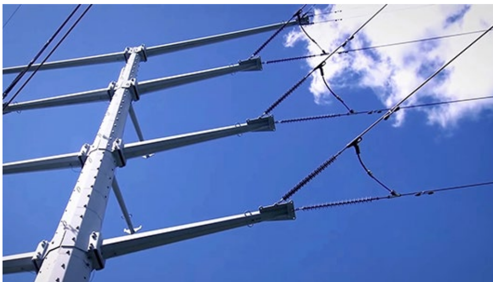
| American Transmission Co.
