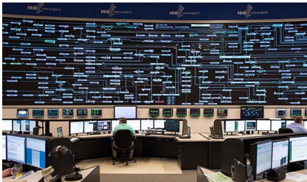
ISO-NE control room | ISO-NE
