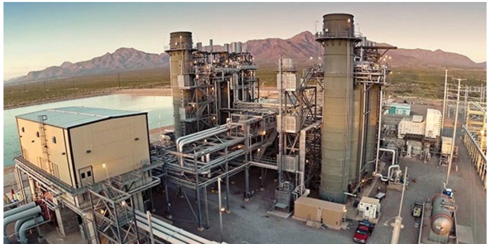
EPE's Newman Generating Station | El Paso Electric
