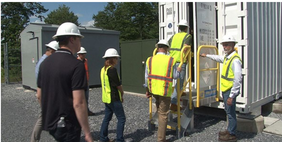
Workers enter a container-size energy storage unit in New York. | NY-BEST
