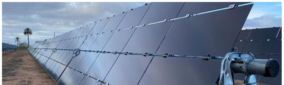
NextEra Energy Resources' Pinal Central Energy Center in Arizona, combining solar with storage | NextEra Energy Resources
