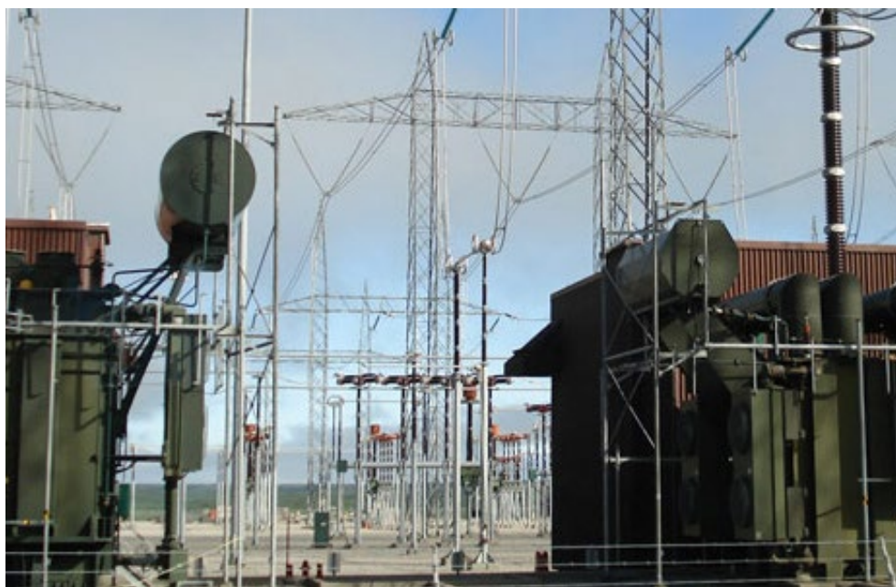
Hydro-Québec transmission substation
