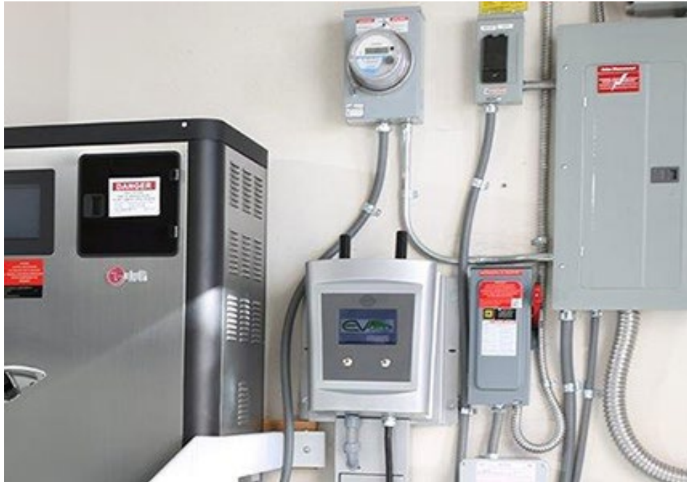
Home battery storage systems are at the heart of the controversy over well backups in the CPUC’s Self Generation Incentive Program. | Southern California Edison
