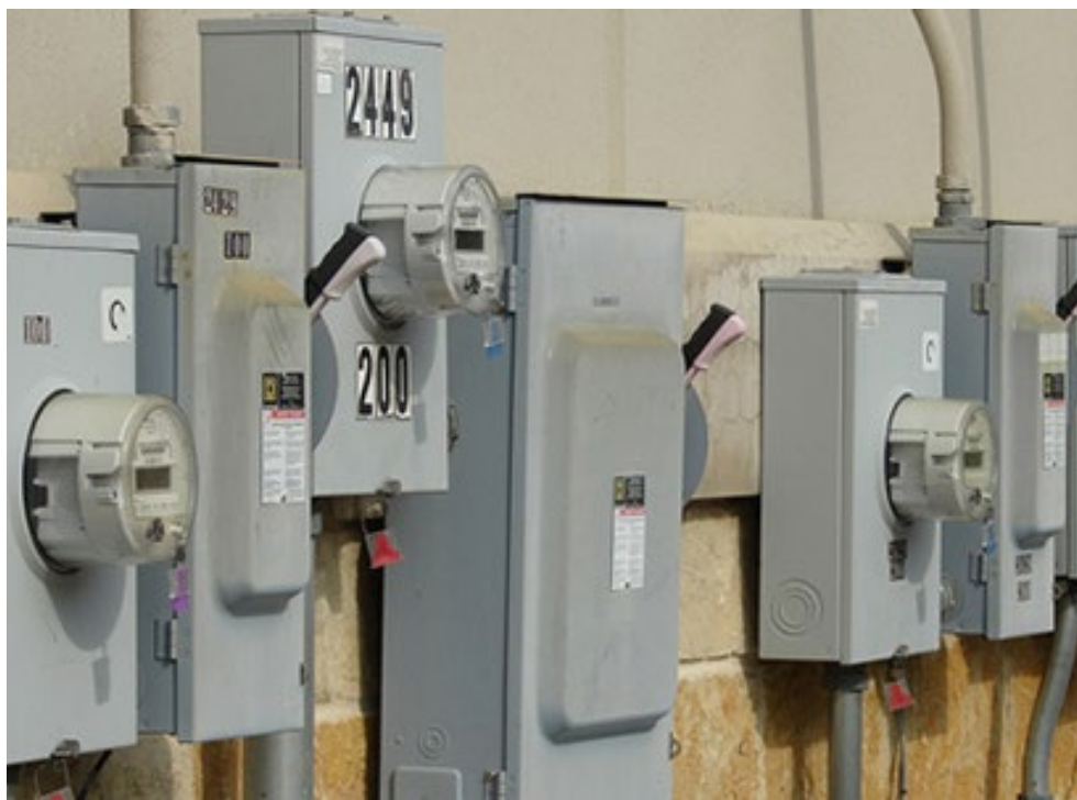
Electric meter boxes
