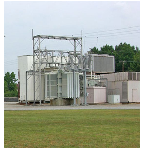
Tasley, a single-unit 33 MW industrial gas turbine that began commercial operation in 1972 in Tasley, Va., is a black start-capable unit. | Calpine
