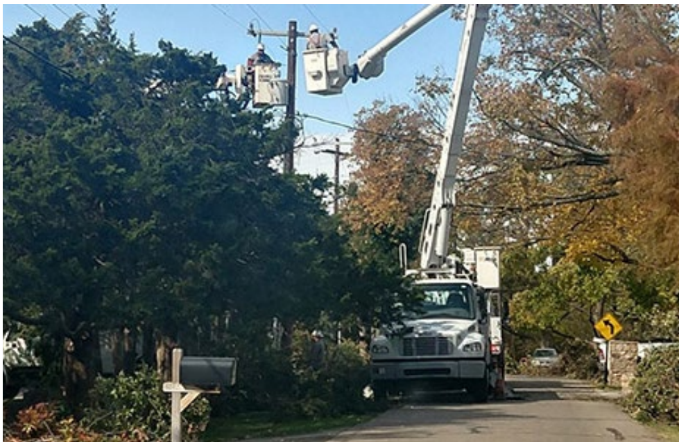
OG&E is still recovering from the worst ice storm in the company's history. | Oklahoma Gas & Electric
