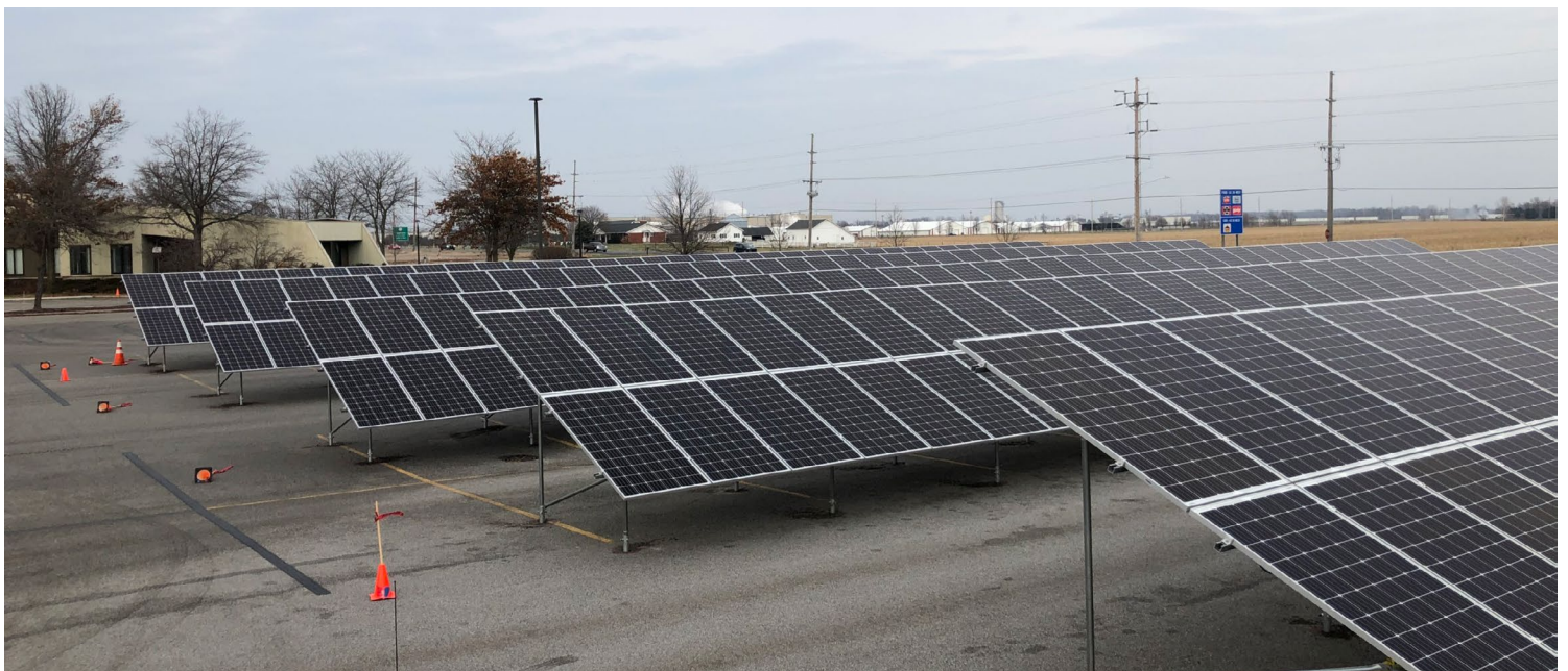
NIPSCO solar array | Inovateus Solar
