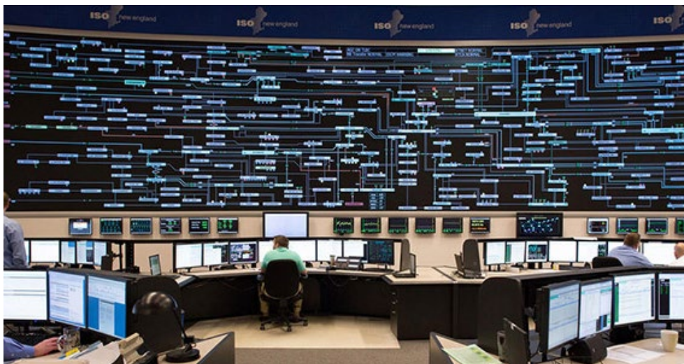
ISO-NE control room | ISO-NE
