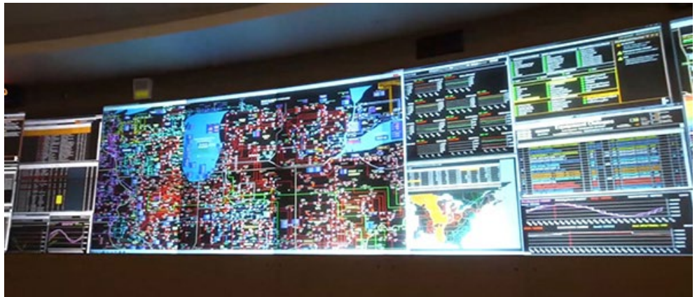
MISO control room | MISO
