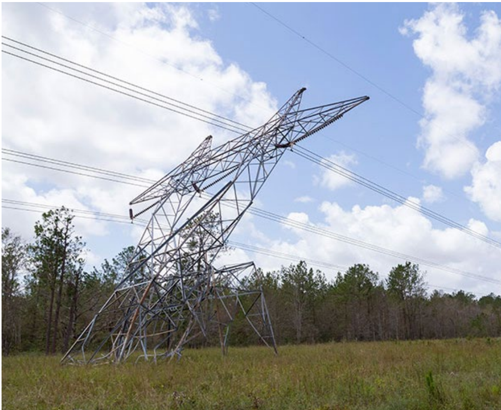
Damaged transmission caused by Hurricane Laura | Entergy
