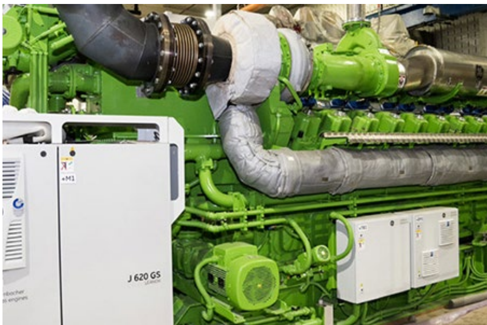
The New York City Department of Environmental Protection is halfway through a $300 million project to install five cleaner-operating cogeneration engines at the North River Wastewater Resource Recovery Facility in West Harlem. | NYC DEP
