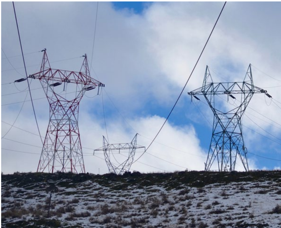
Pacific DC Intertie at The Dalles | © RTO Insider
