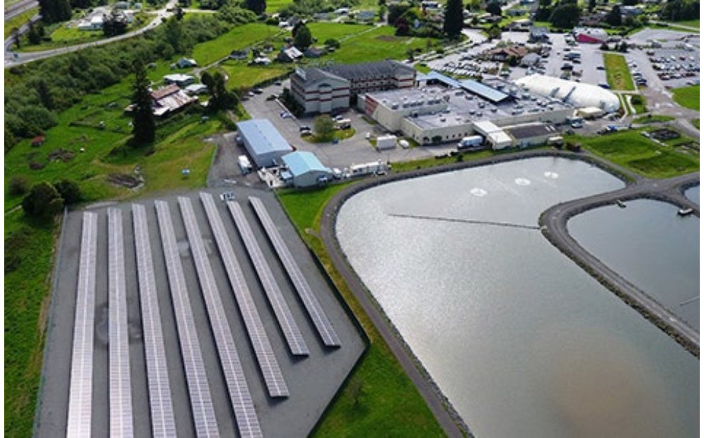
The Blue Lake Rancheria in Humboldt County installed a microgrid to provide power during PSPS. | Siemens
