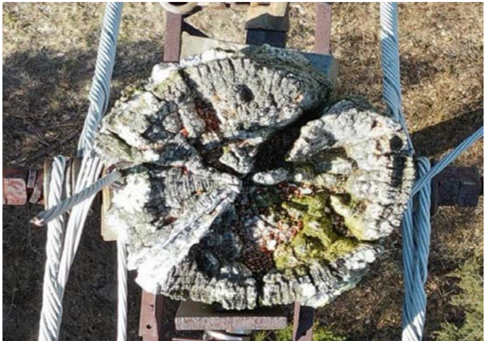
An example of pole top rot from Connecticut | Eversource
