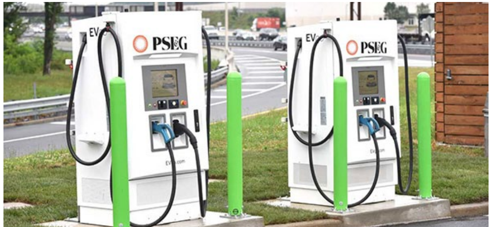
Two EVgo 480-V fast chargers at the Molly Pitcher Service Area on the New Jersey Turnpike. The chargers can provide 150 miles of range per hour. | PSE&G
