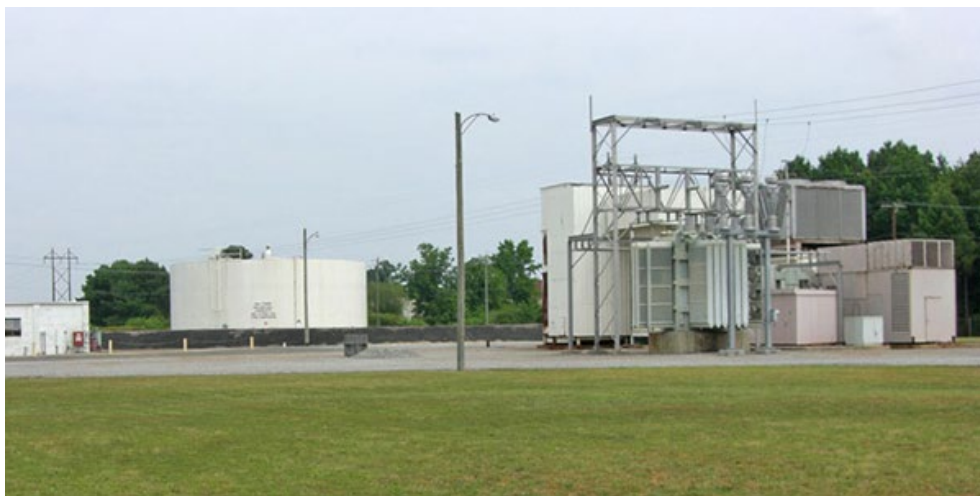
Tasley, a single-unit 33 MW industrial gas turbine that began commercial operation in 1972 in Tasley, Va., is a black start-capable unit. | Calpine
