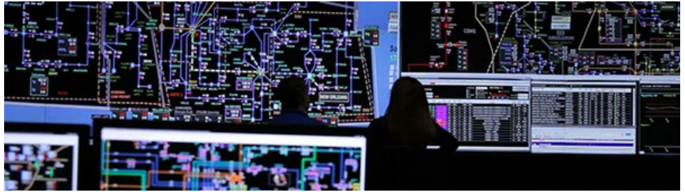
MISO control room | MISO
