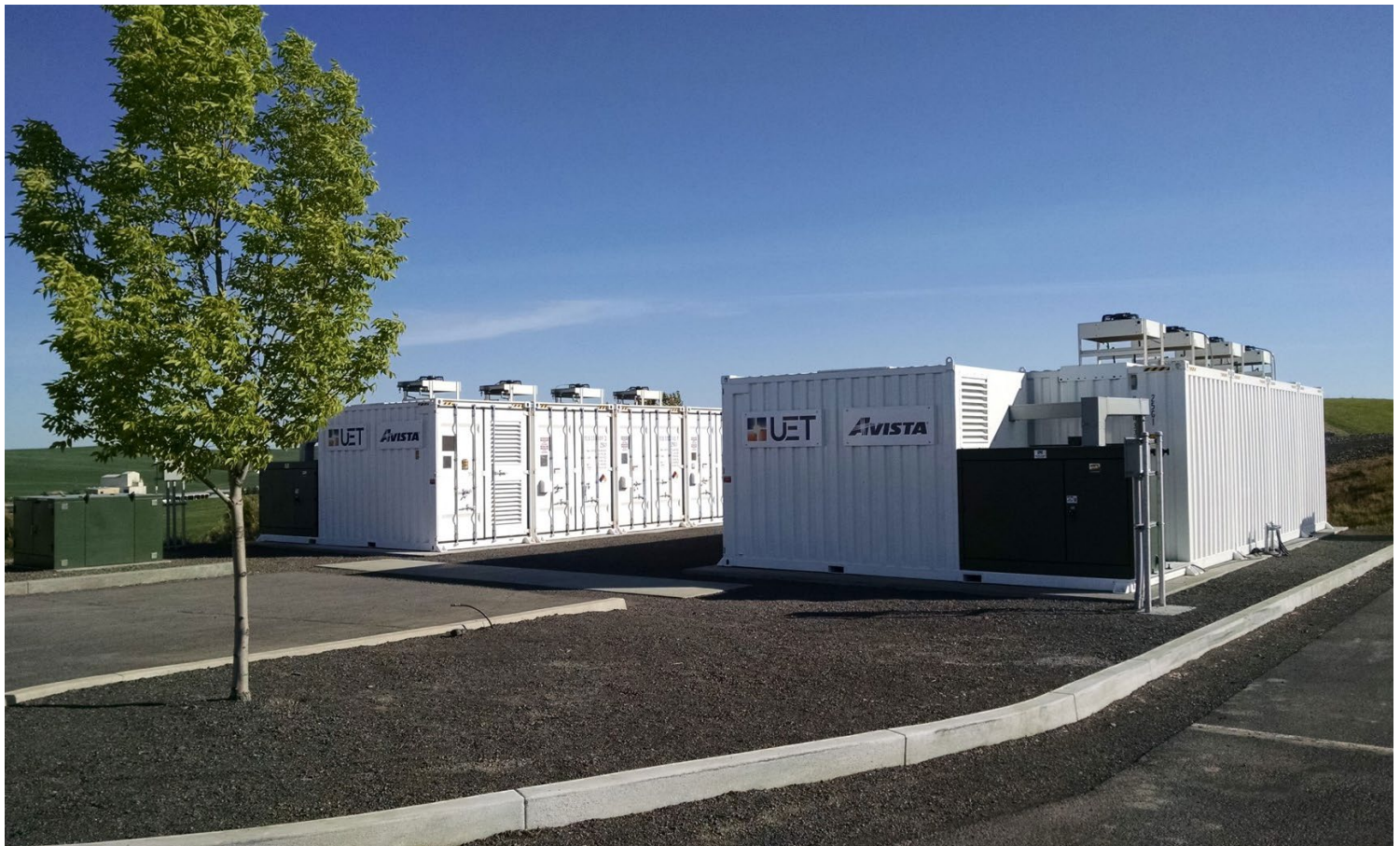
Avista's Turner Energy Storage Project in Pullman, Wash. | UniEnergy Technologies, CC-BY-SA-4.0 via Wikimedia Commons
