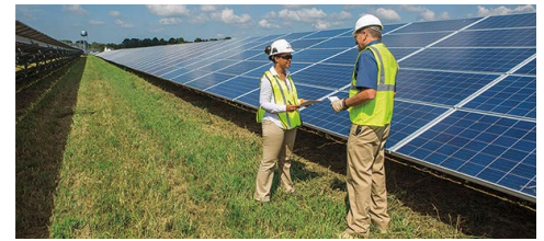
Dominion Energy solar farm in Louisa County, Va. | Dominion Energy
