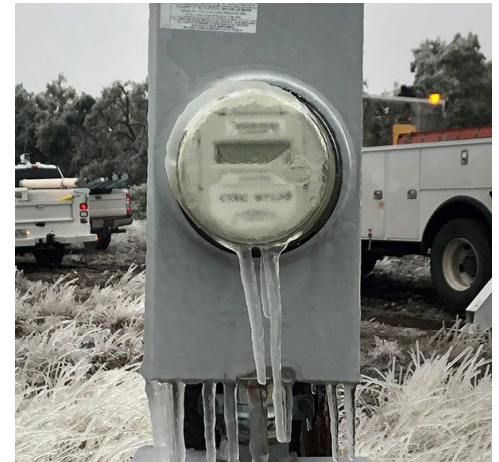
Iced meter in Texas | Kerrville Public Utilities Board
