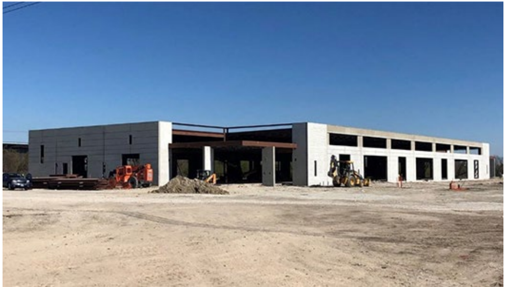
ERCOT's new headquarters facility is being built close to its current location in Austin. | ERCOT
