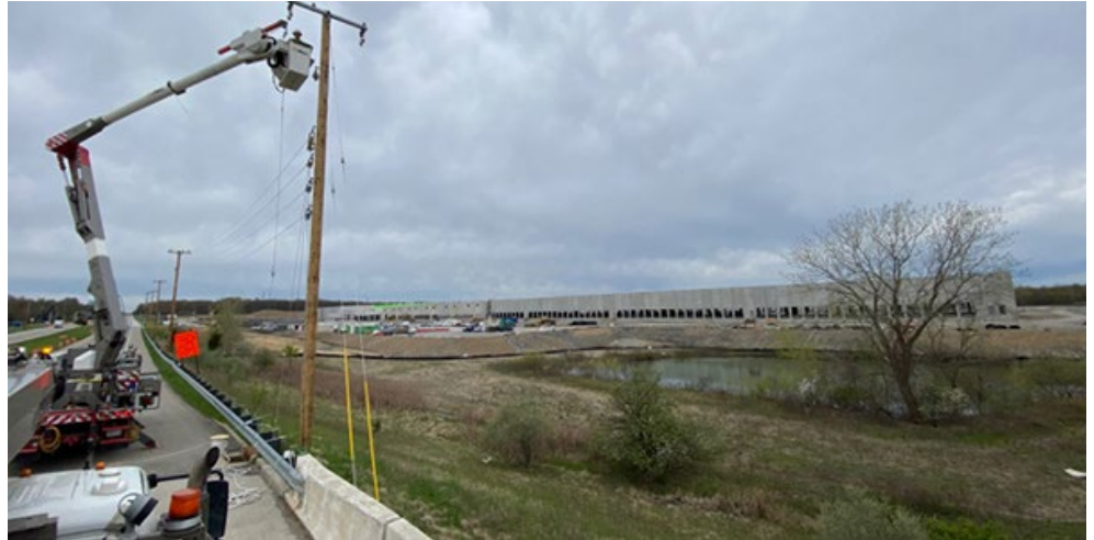
FirstEnergy has started construction on a new transmission substation in Trumbull County, Ohio, to support the expanding electric vehicle industry in the region. | FirstEnergy
