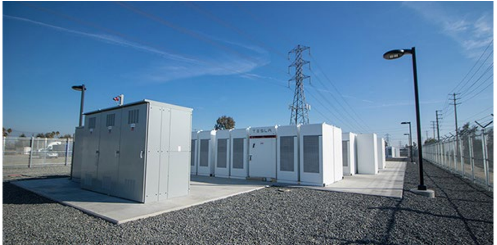
Making sure battery storage can function well as an RA resource is among the CAISO initiative's goals. | Southern California Edison
