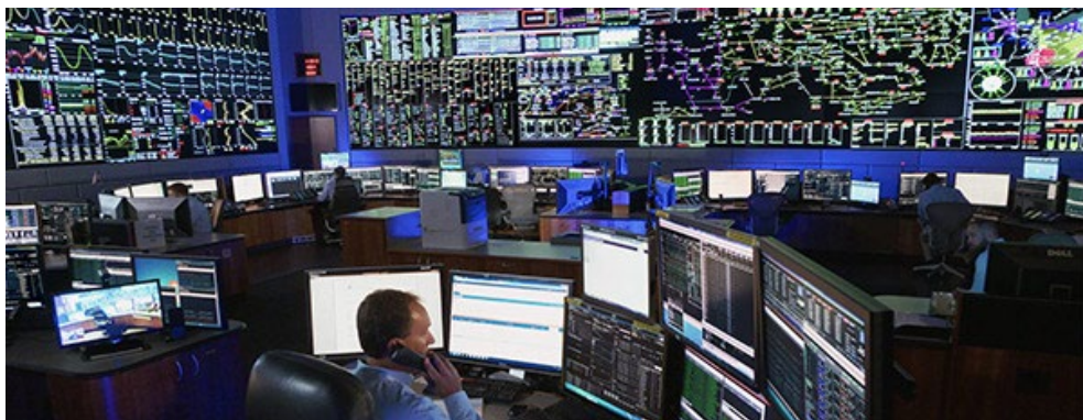
PJM control room | PJM
