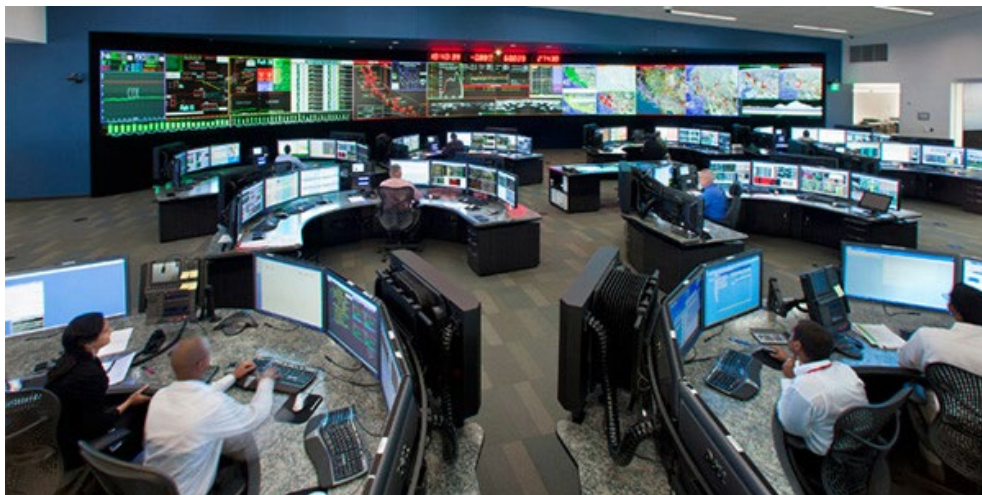
CAISO's control room in Folsom, Calif. | CAISO
