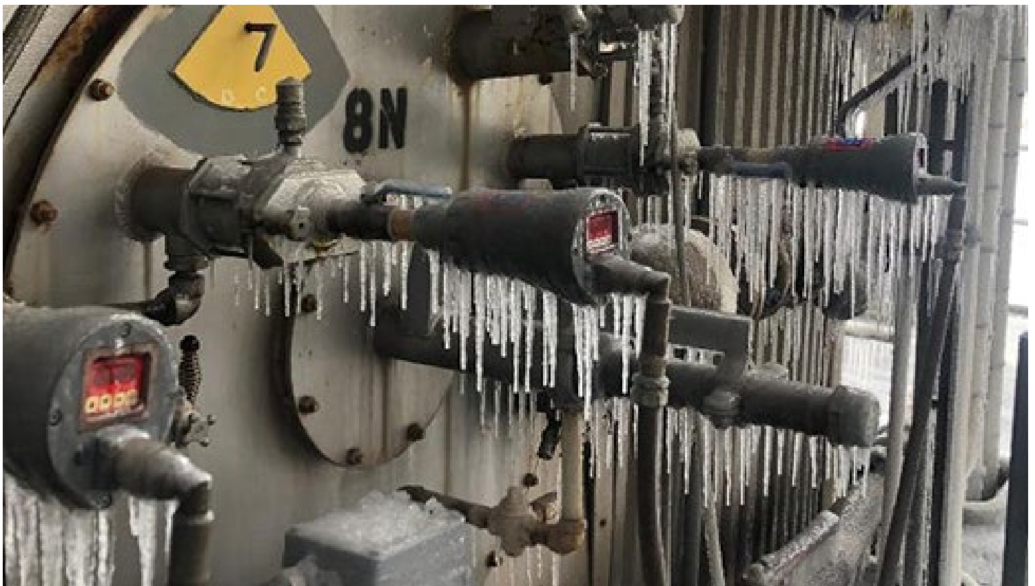
Frozen instrumentation on a power plant | Entergy
