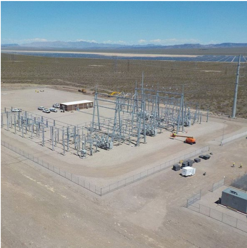
GridLiance's Sloan Canyon Switching Station near Hoover Dam in Nevada | GridLiance
