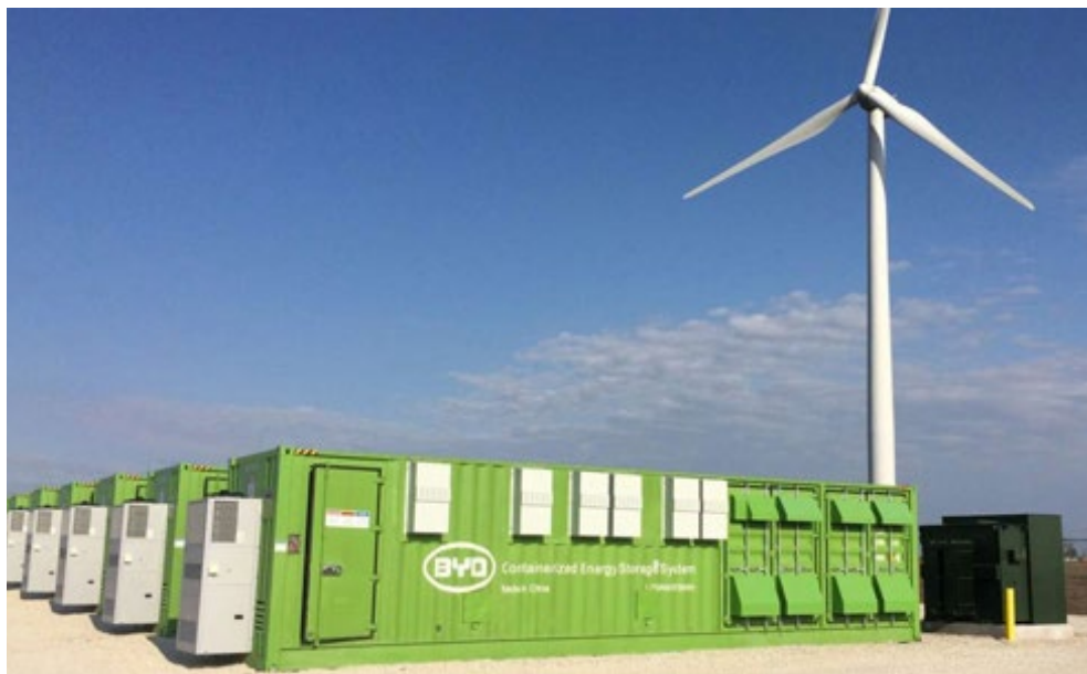
Invenery's Grand Ridge Battery Storage Facility in Illinois | BYD
