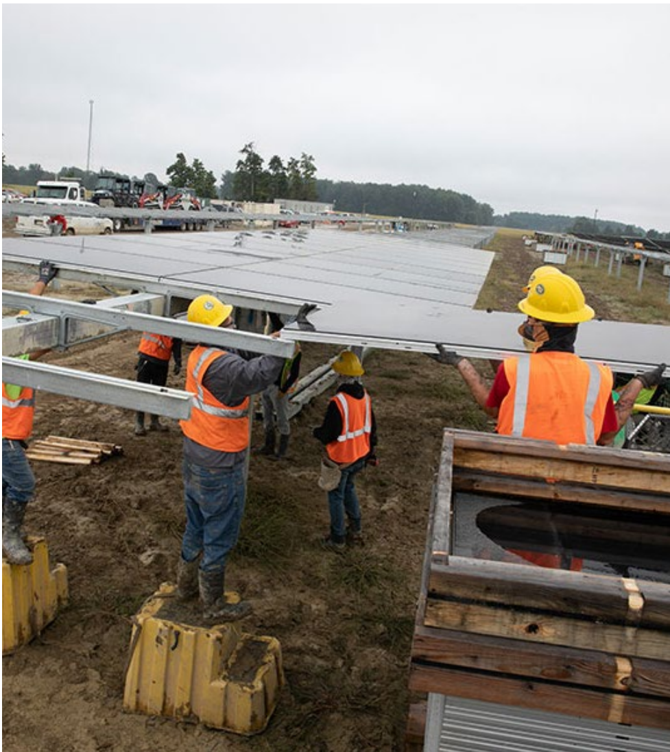
Innergex Renewables Development USA has nearly completed the 200-MW Hillcrest Solar Project in Brown County in southwest Ohio. Innergex will pay a total of $1.8 million annually to the Western Brown Local School District, Green Township and Brown County for the next 35 years. | Innergex Renewables Development USA
