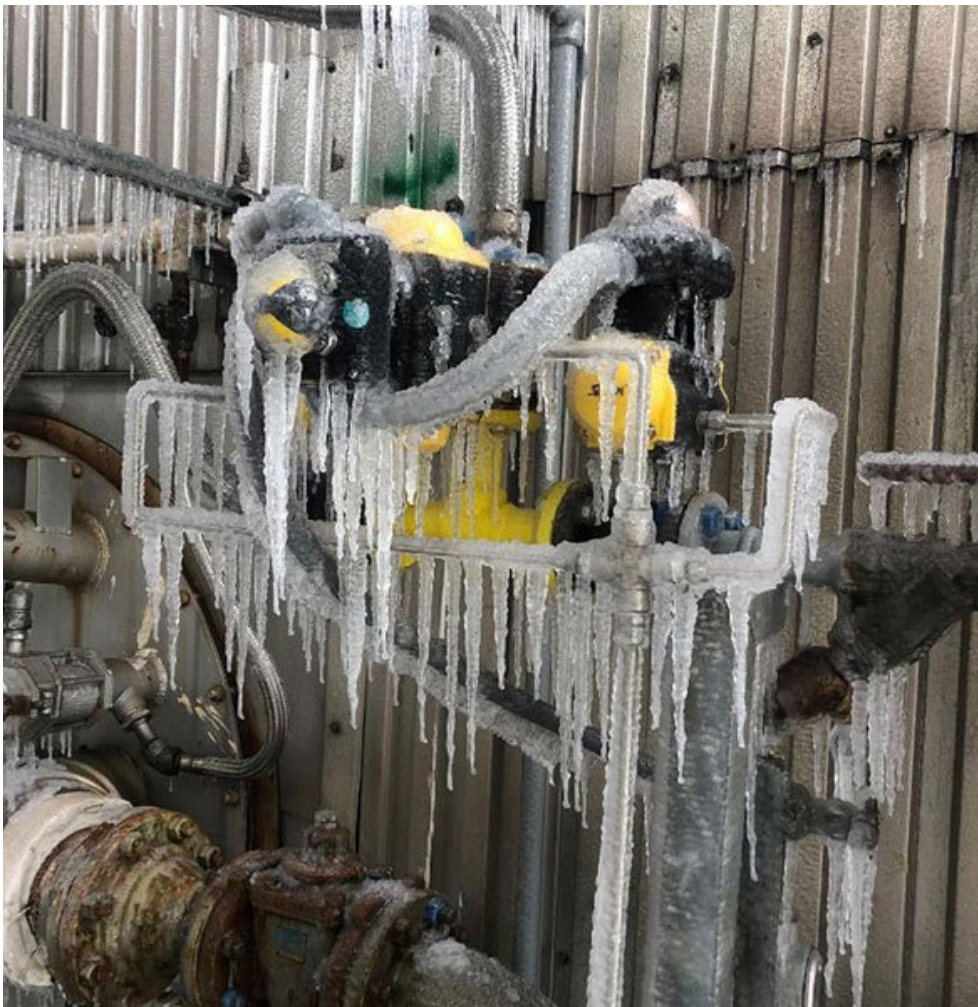
Frozen equipment at an Entergy power plant | Entergy
