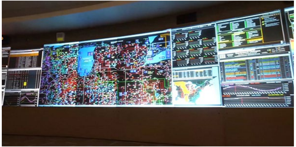
MISO control room | MISO
