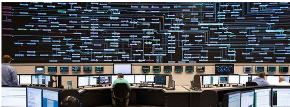
ISO-NE control room | ISO-NE
