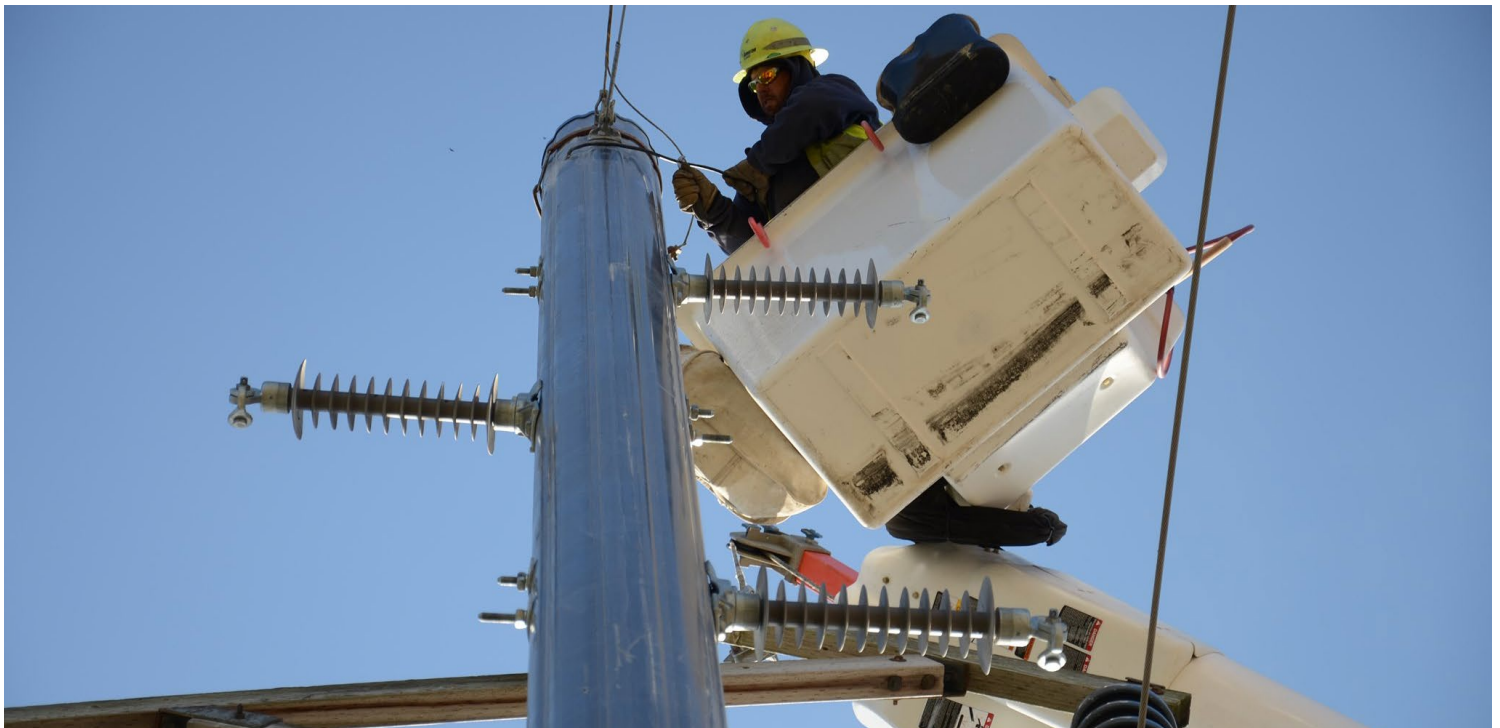
An Ameren Illinois worker upgrading poles to better withstand wind and ice accumulations | Ameren Illinois
