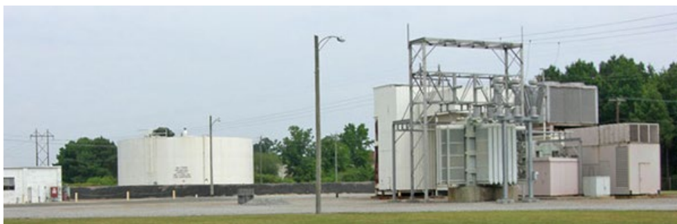
Tasley, a single-unit 33 MW industrial gas turbine that began commercial operation in 1972 in Tasley, Va., is a black start-capable unit. | Calpine
