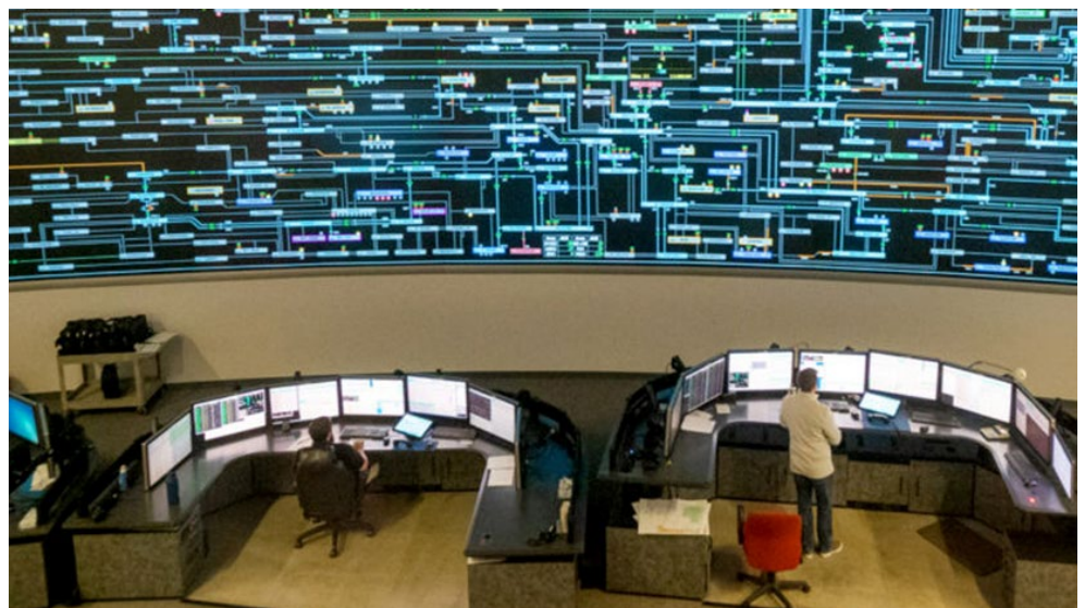
ISO-NE control room | ISO-NE
