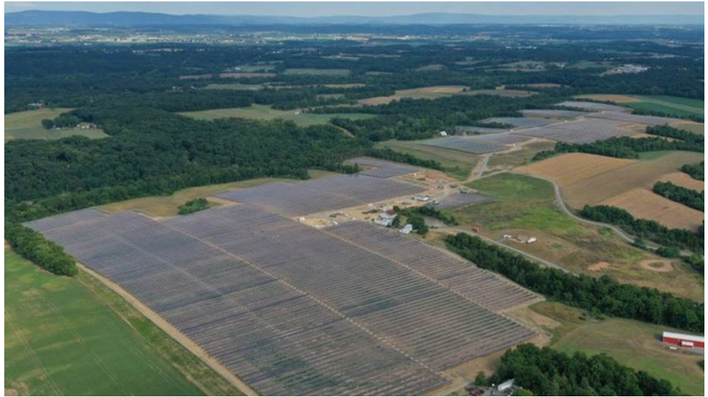
One of three solar farms that make up the 70-MW solar array in Franklin County, Pa., that will provide Penn State with 25% of its purchased electricity, across all campuses, over 25 years | Lightsource bp
