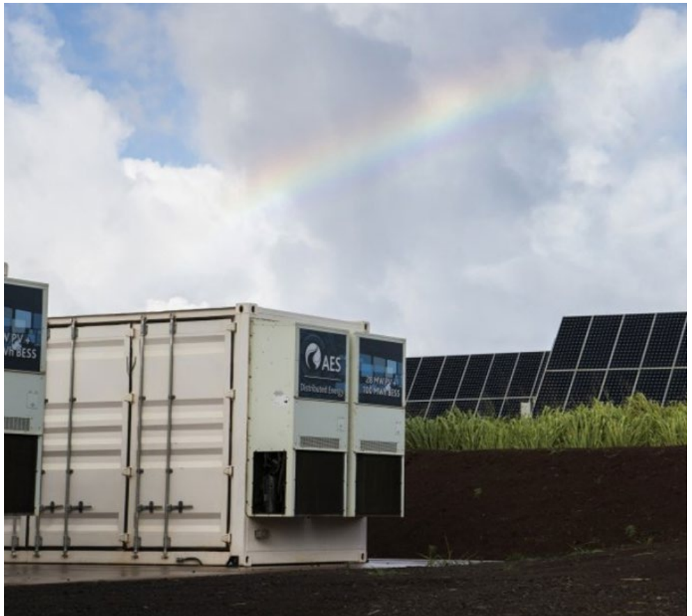
Understanding the variety of interconnection rules across jurisdictions is a significant challenge for developers of hybrid storage projects, like solar paired with batteries. | National Renewable Energy Laboratory
