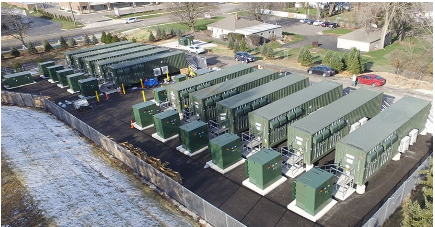
EDF Renewables' McHenry storage project in Illinois | EDF Renewables
