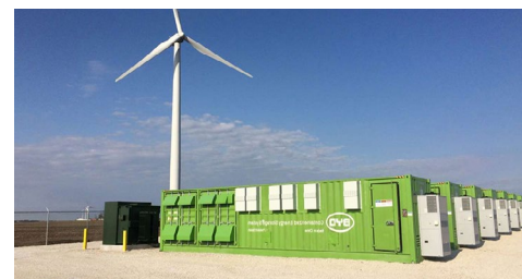
Invenergy's Grand Ridge Battery Storage Facility | BYD
