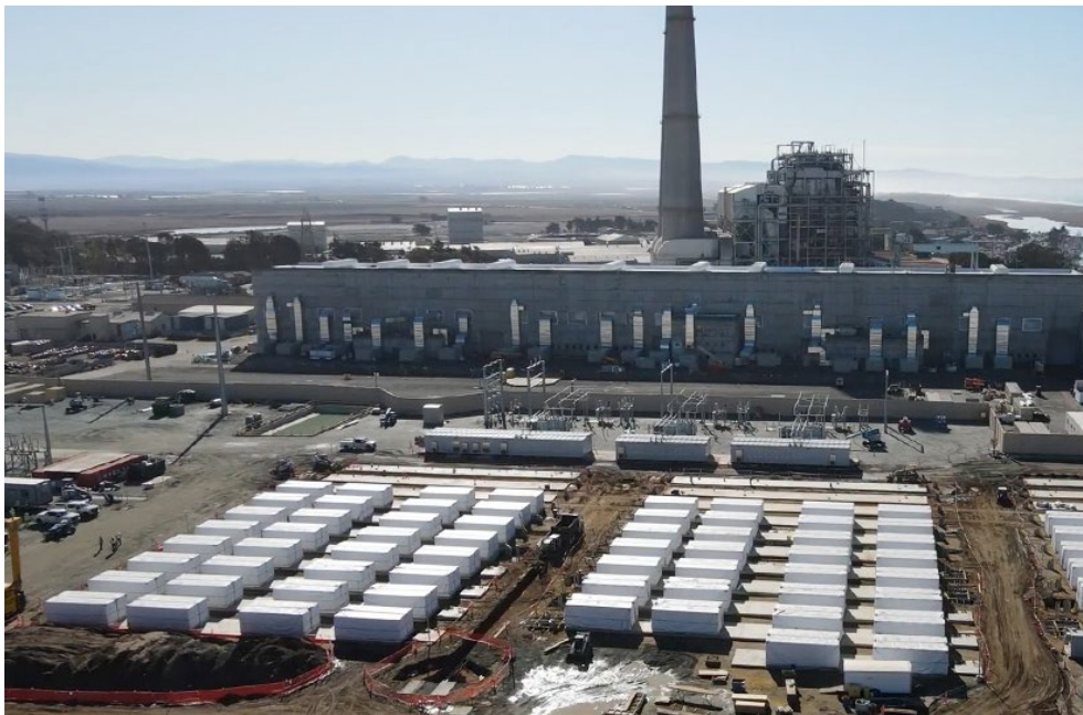
PG&E and Tesla are building one of the nation's largest storage facilities at the utility's old Moss Landing power plant on Monterey Bay. | EKM Metering
