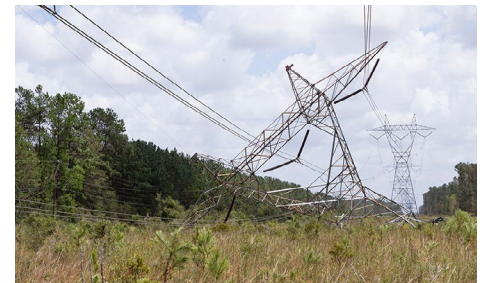
Transmission tower damaged by Hurricane Laura | Entergy
