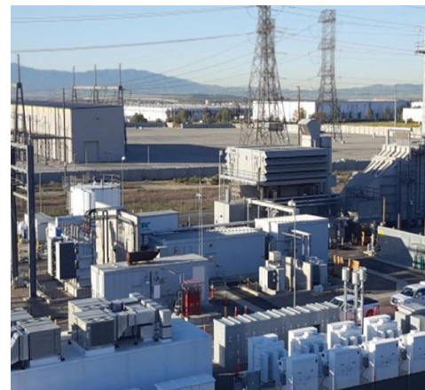
Southern California Edison’s Grapeland Peaker in Rancho Cucamonga | Southern California Edison, via Wellhead Power Solutions
