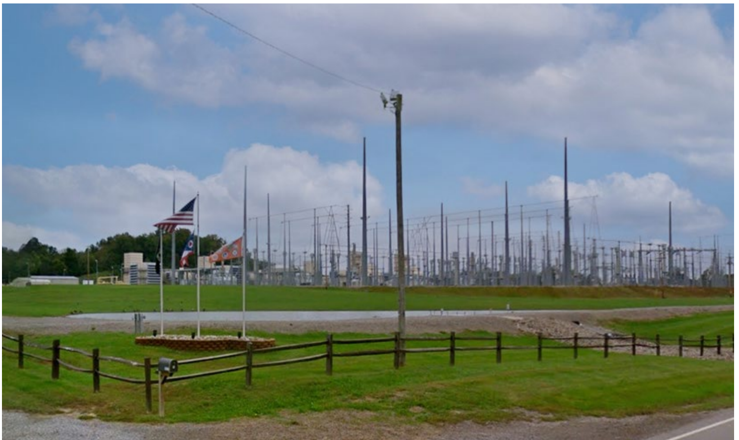
Eastern Generation is upgrading its 850-MW Rolling Hills natural gas generator in Vinton County, Ohio, by 90 MW. | Google
