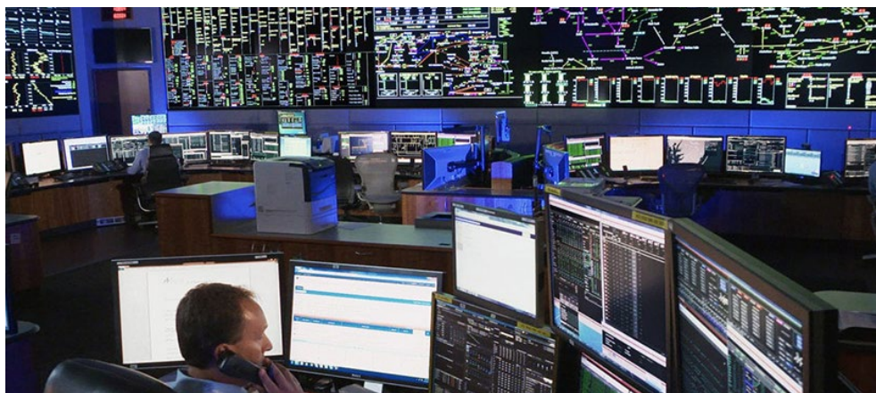
PJM control room. | PJM
