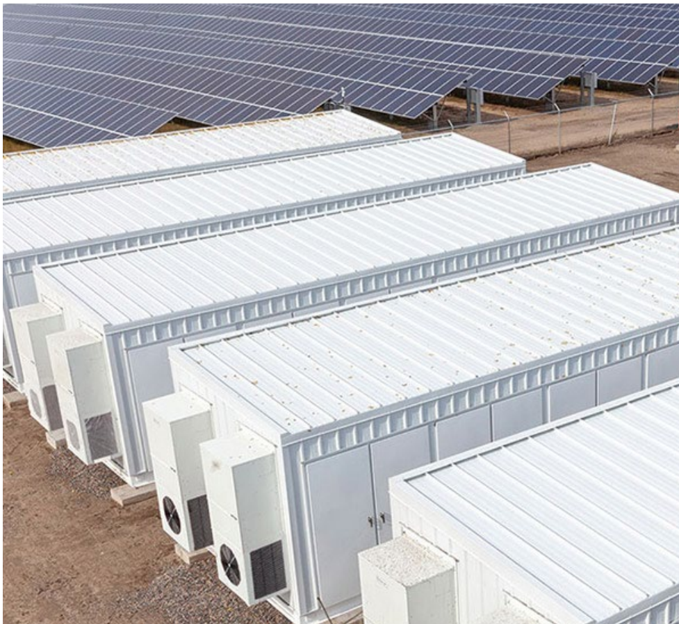
Energy storage in Minnesota | Connexus Energy
