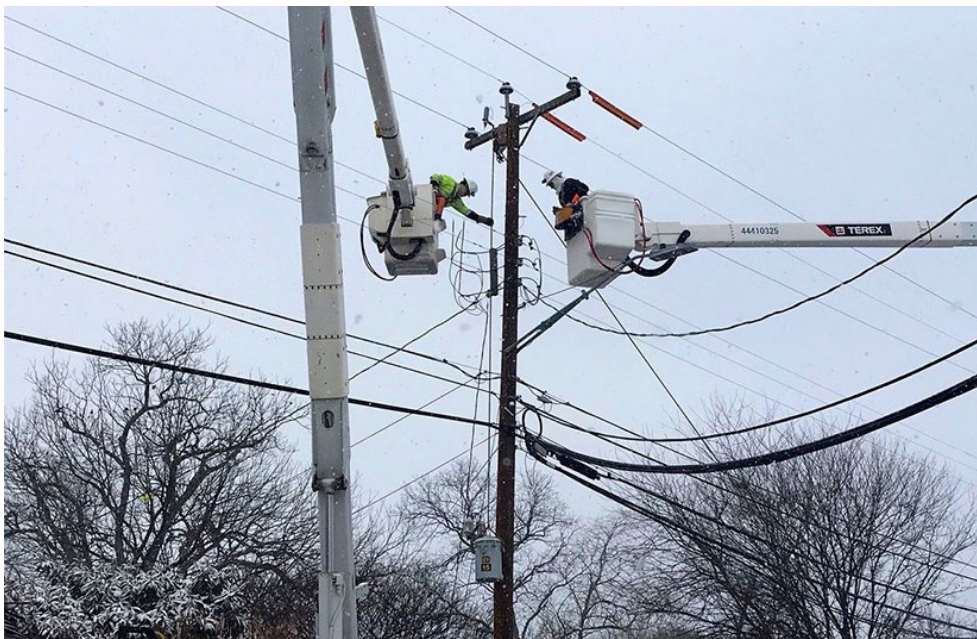
A CPS Energy crew works to restore power following the February winter storm. | CPS Energy
