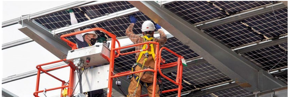
Workers in Vermont install a solar awning that will support the state's energy plan of meeting 90% of its energy needs from renewables by 2050. | SunCommon
