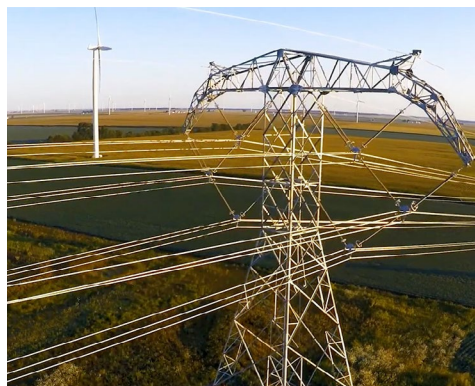
AEP owns the nation's largest electric transmission system, totaling more than 40,000 miles. | AEP
