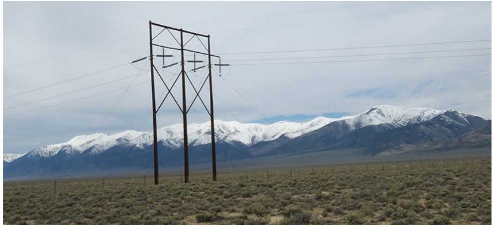
Long distance high-voltage lines are planned for Nevada, Wyoming, Utah and Colorado. | © RTO Insider LLC
