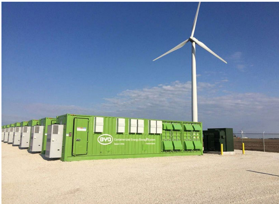
Invenergy's Grand Ridge Battery Storage Facility | BYD
