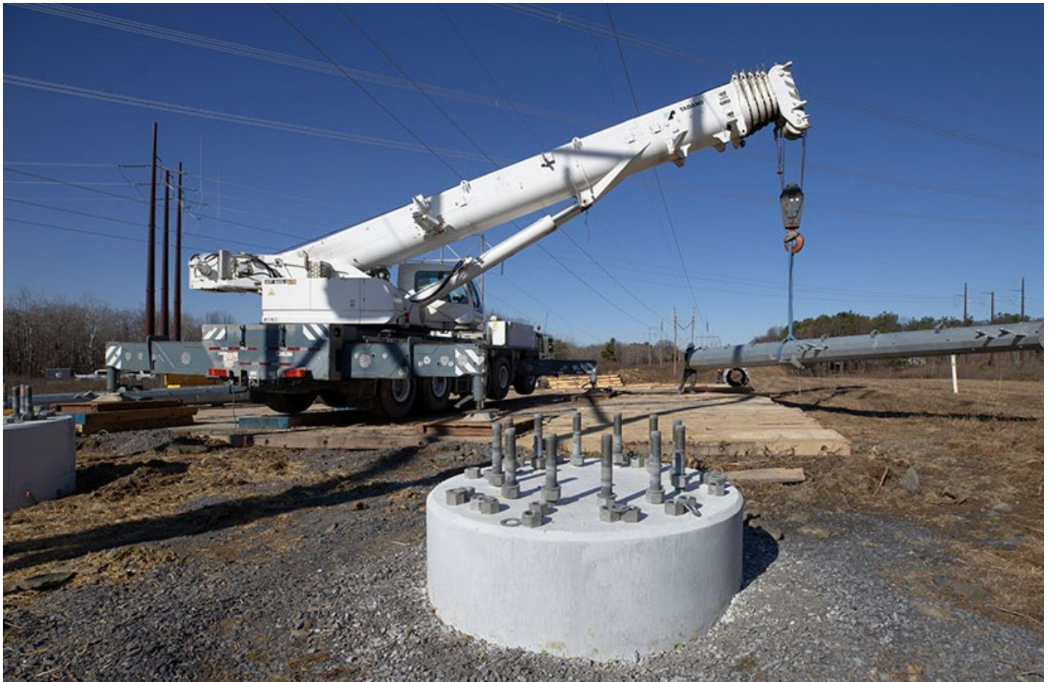
A crew in March 2021 raises a transmission pole on the Marcy to New Scotland Transmission Upgrade Project. | NYPA
