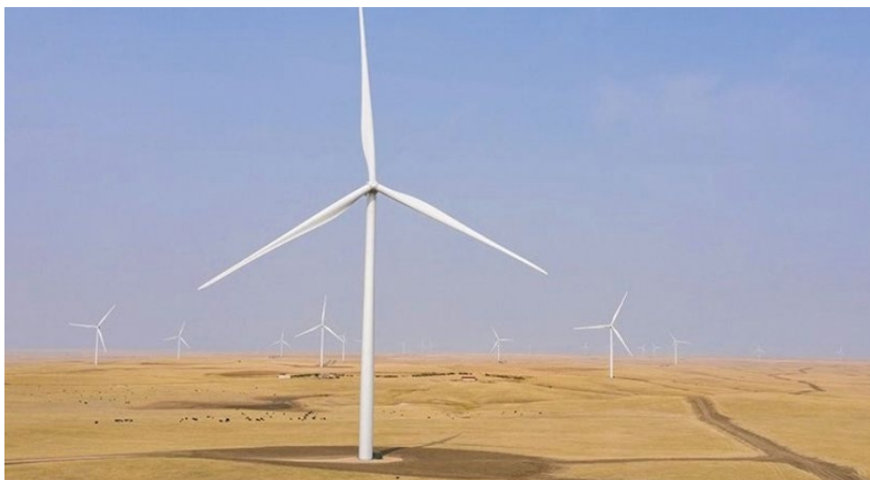
Proposals to build stable renewable energy tax credits for projects like the Willow Creek Wind farm would allow renewables to develop at the pace needed to meet the Biden administration’s climate goals. | Ørsted U.S.
