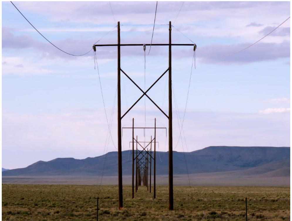
NV Energy, the main transmission owner in Nevada, could benefit from being in an RTO, the PUCN said. | © RTO Insider LLC
