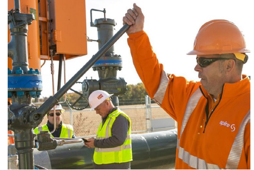
The Spire STL Pipeline went into commercial operation in November 2019. | Spire
