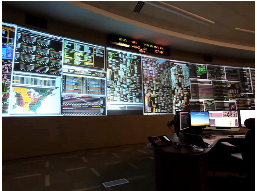
MISO control room | MISO
