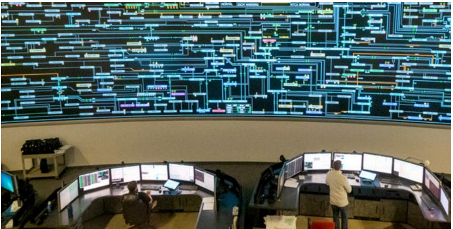
ISO-NE control room | ISO-NE
