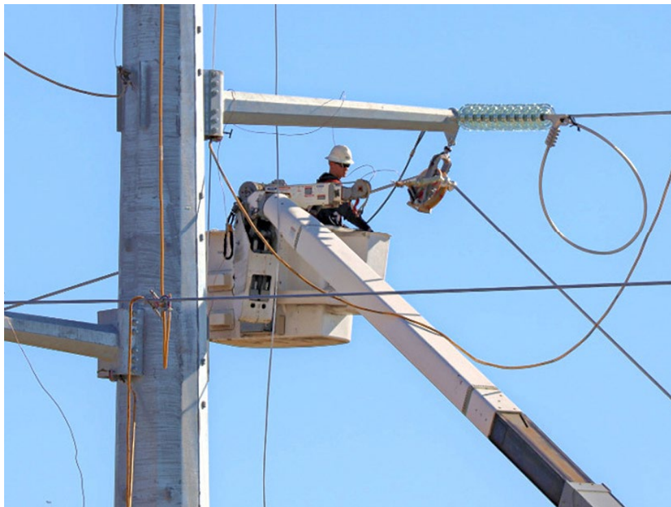
A FirstEnergy employee works on a transmission line in northern Ohio in 2020. | FirstEnergy
