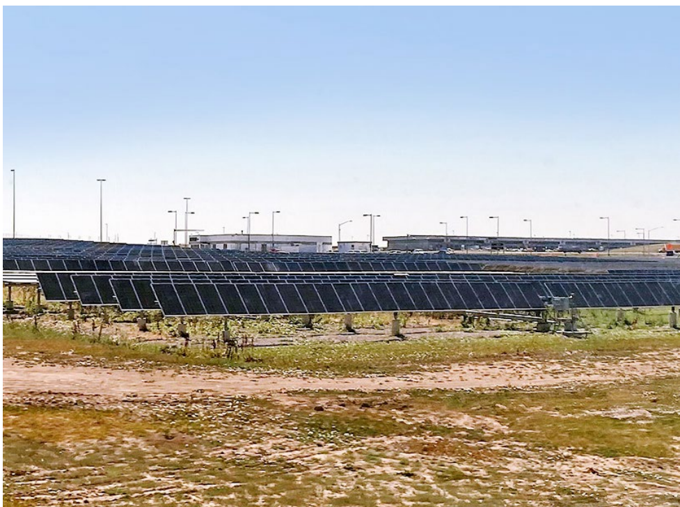
Solar installations at Denver International Airport greeted attendees of NARUC's Summer Policy Summit. | © RTO Insider LLC
