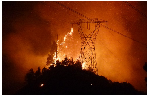
A wildfire burned near high-voltage lines in south-central Washington state in 2013. | Washington State Department of Transportation
