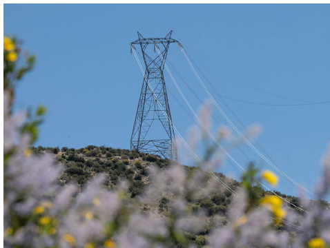
Insulated lines run above an arid, fire-prone landscape in SCE's service territory. | Elisa Ferrari/SCE
