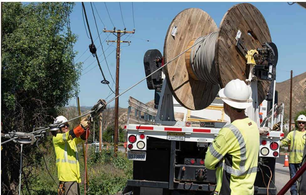
Workers unspool covered conductor as part of Southern California Edison's grid hardening efforts against wildfires. | Elisa Ferrari/SCE
