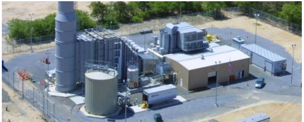
NYPA is studying the effects of blending green hydrogen with natural gas at its Brentwood peaker plant on Long Island. | NYPA
