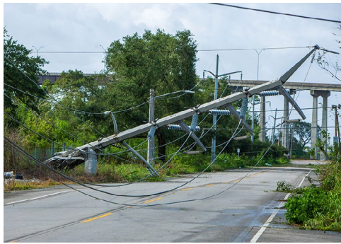
Downed transmission line in New Orleans | Entergy
