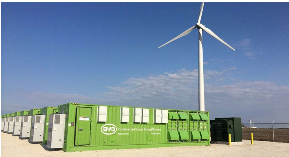
Invenergy's Grand Ridge Battery Storage Facility | BYD
