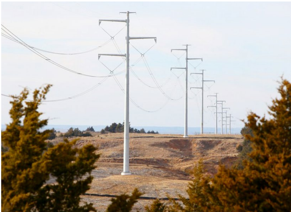
Oklahoma Gas and Electric's 121-mile Windspeed transmission line | Oklahoma Gas and Electric
