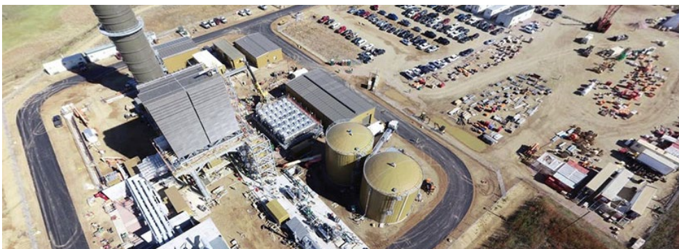
Otter Tail Power Co.'s new Astoria natural gas plant in South Dakota | Otter Tail Power Co.
