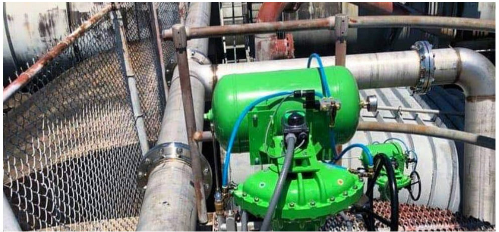
Drainage pumps | New Orleans Sewerage and Water Board
