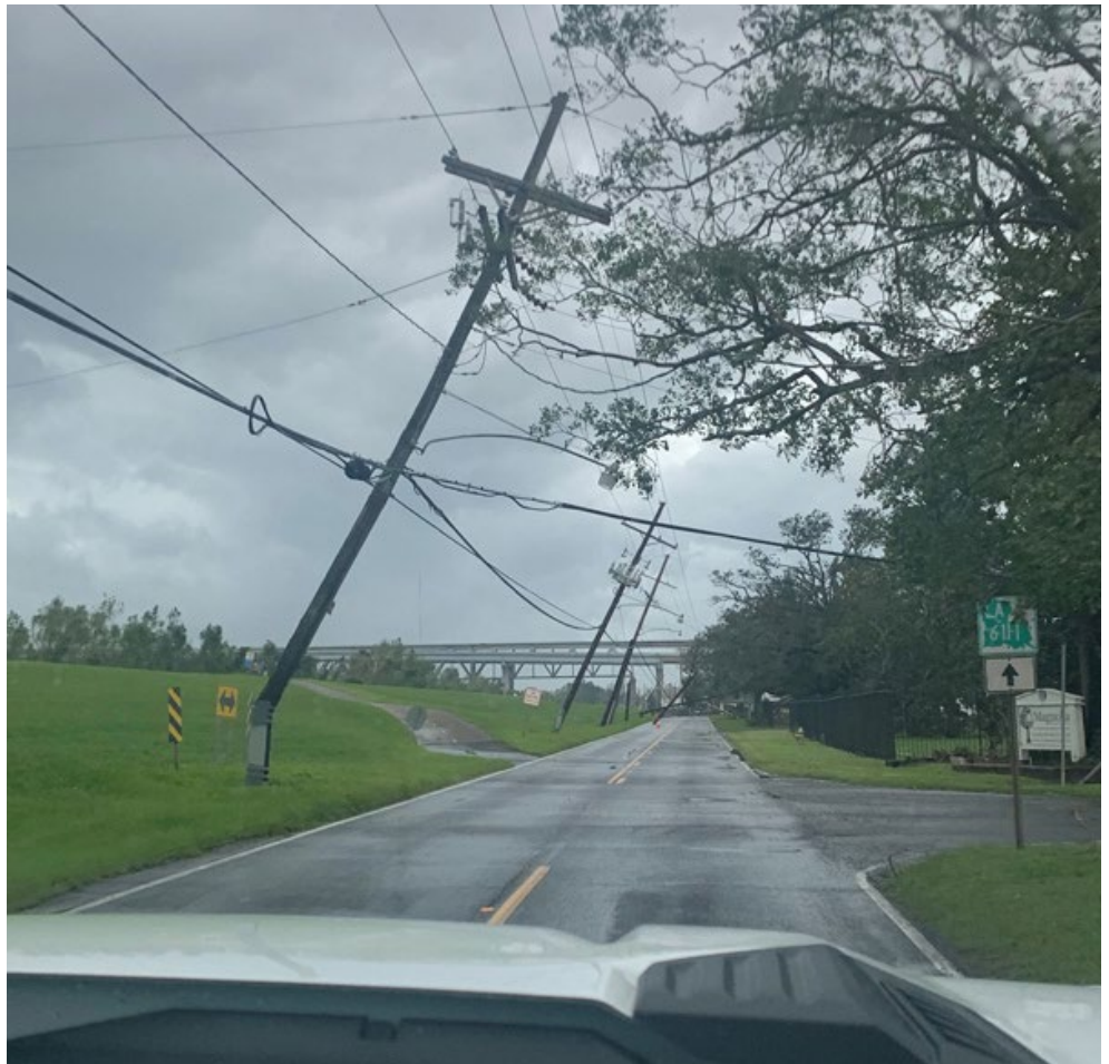
Distribution lines tilt perilously at the border of Metairie and Kenner, La. | Entergy
