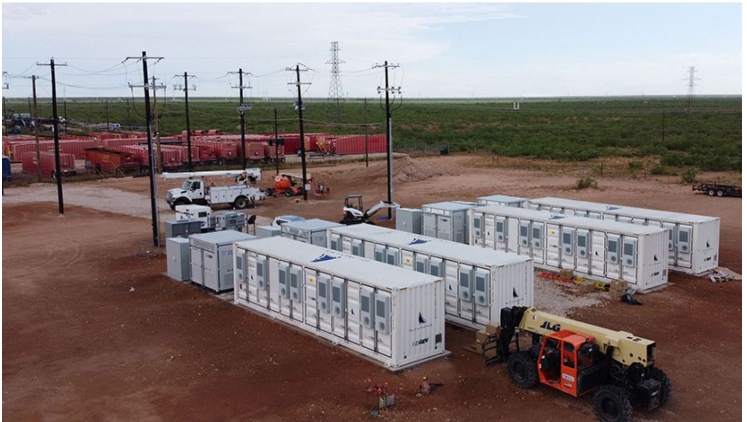
ERCOT is expecting more than 600 MW of energy storage, similar to Broad Reach Power's Odessa project in West Texas, to provide mostly ancillary services this fall. | Broad Reach Power
