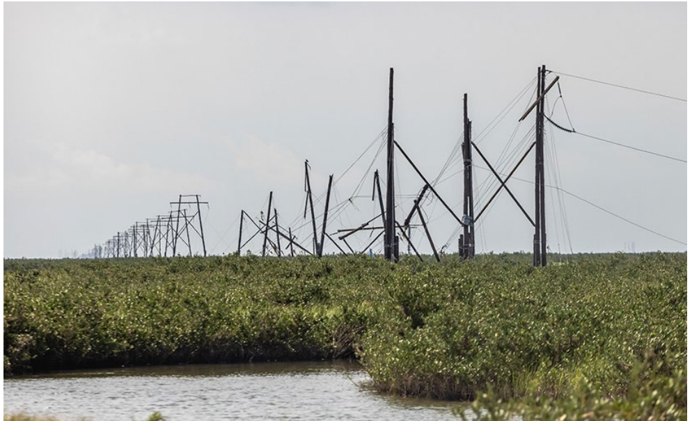
Hurricane Ida destruction in Grand Isle, La. | Entergy
