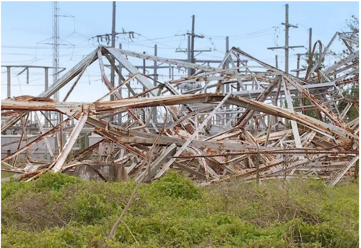
Entergy's fallen transmission tower shows considerable rust. | WWL-TV
