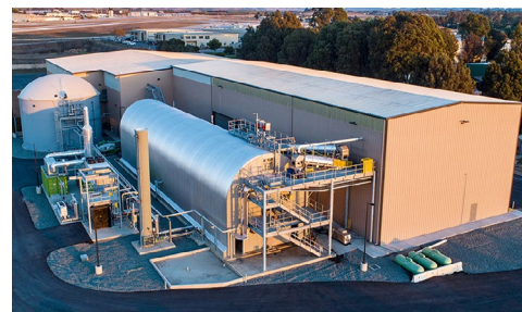
An anaerobic digestion plant in San Luis Obispo, Calif., produces RNG from food and green waste. | Hitachi Zosen Inova
