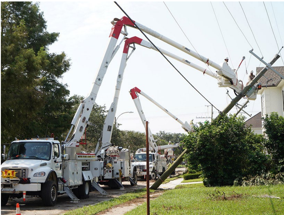
Some 21,000 utility workers are helping to restore power in Louisiana in the wake of Hurricane Ida. | Entergy
