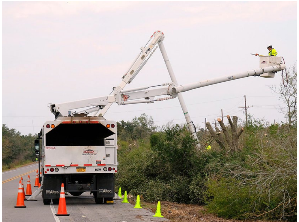
Entergy crews work to restore power in New Orleans. The utility said Sept. 6 that more than half of the 902,000 customers who lost power in Louisiana following Hurricane Ida had been restored. | Entergy
