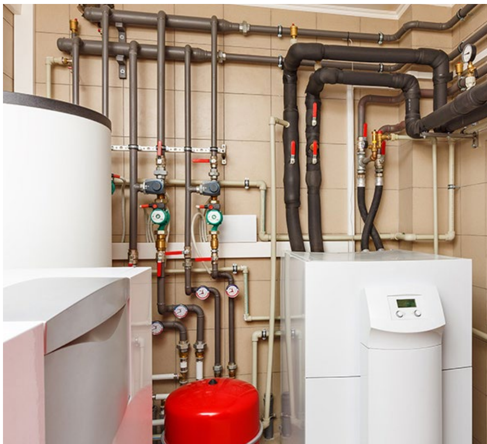
As an alternative to hydrogen, the GeoBlock allows building heat pumps, like the one seen here, to pull heating or cooling off a geothermal supply loop installed in existing natural gas rights-of-way. | Shutterstock
