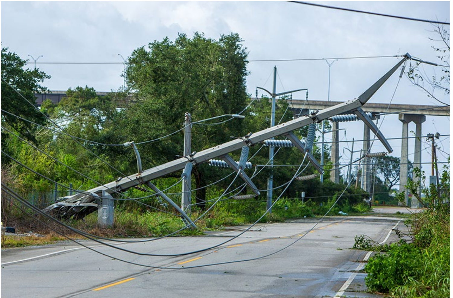
Hurricane Ida damage in New Orleans on Aug. 30 | Entergy
