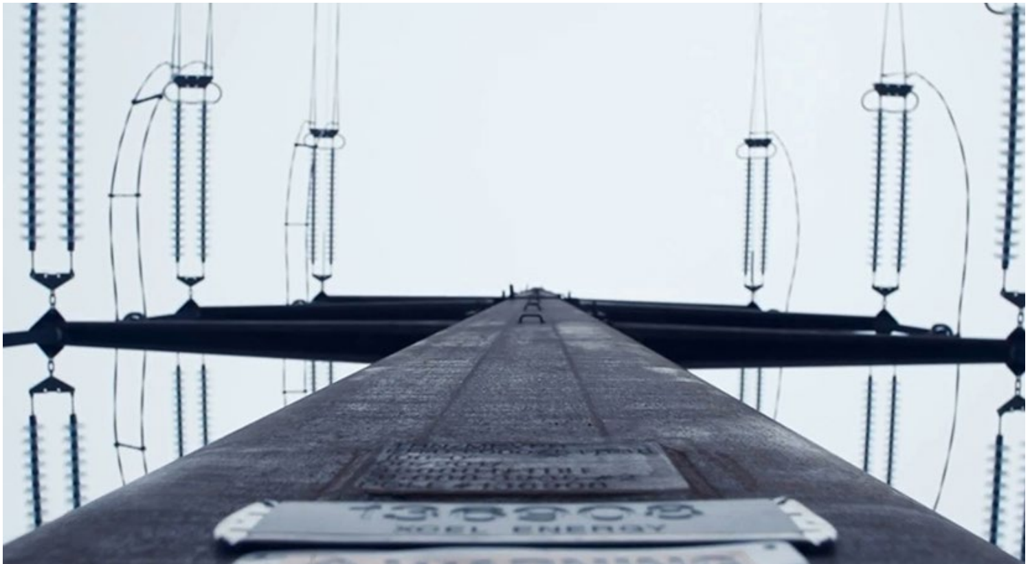
Tower from the Badger-Coulee MVP project in Wisconsin | IBEW
