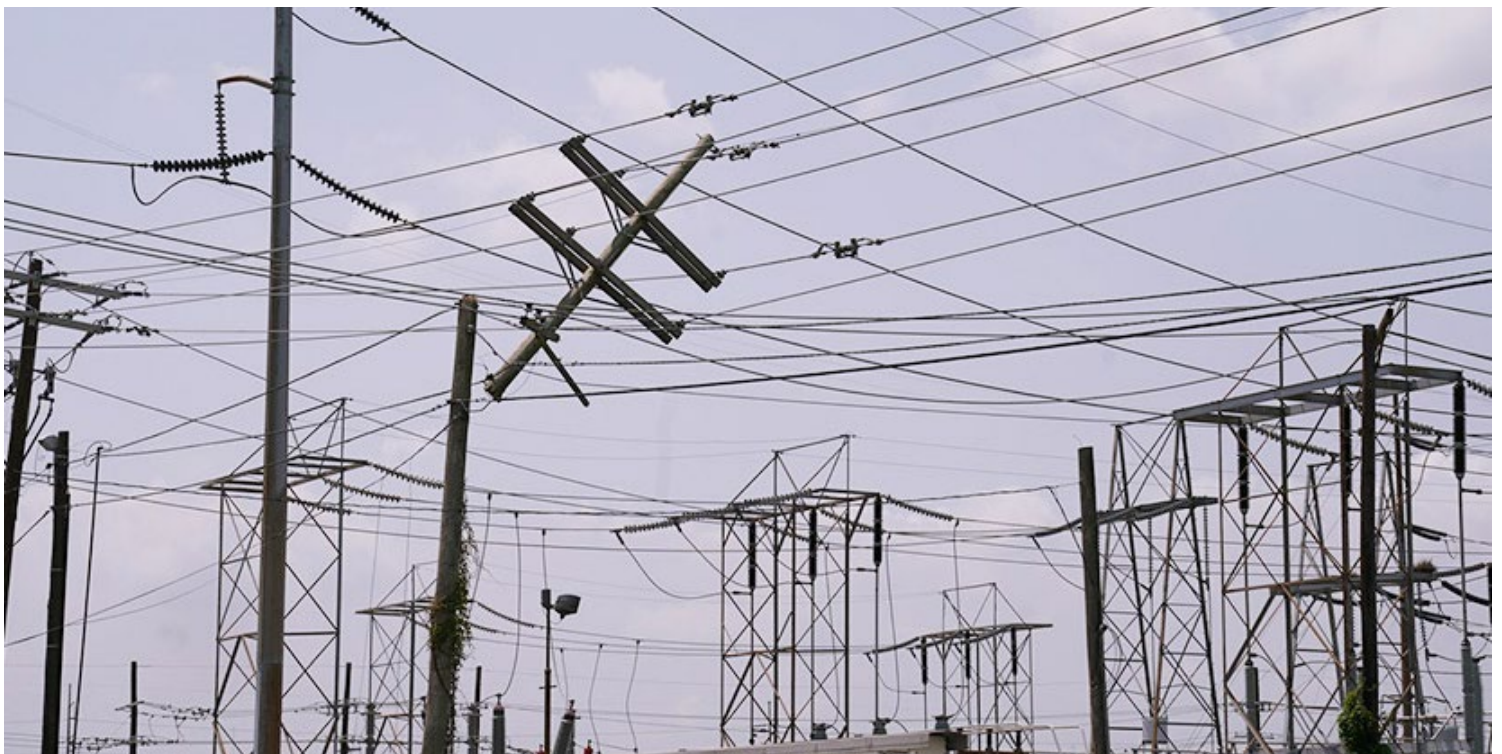
Hurricane Ida damage | Entergy
