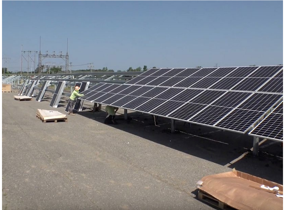
A solar array being installed on the SUNY Fredonia campus, for which the distribution utility, National Grid, will credit the school for all electricity produced. | NYPA
