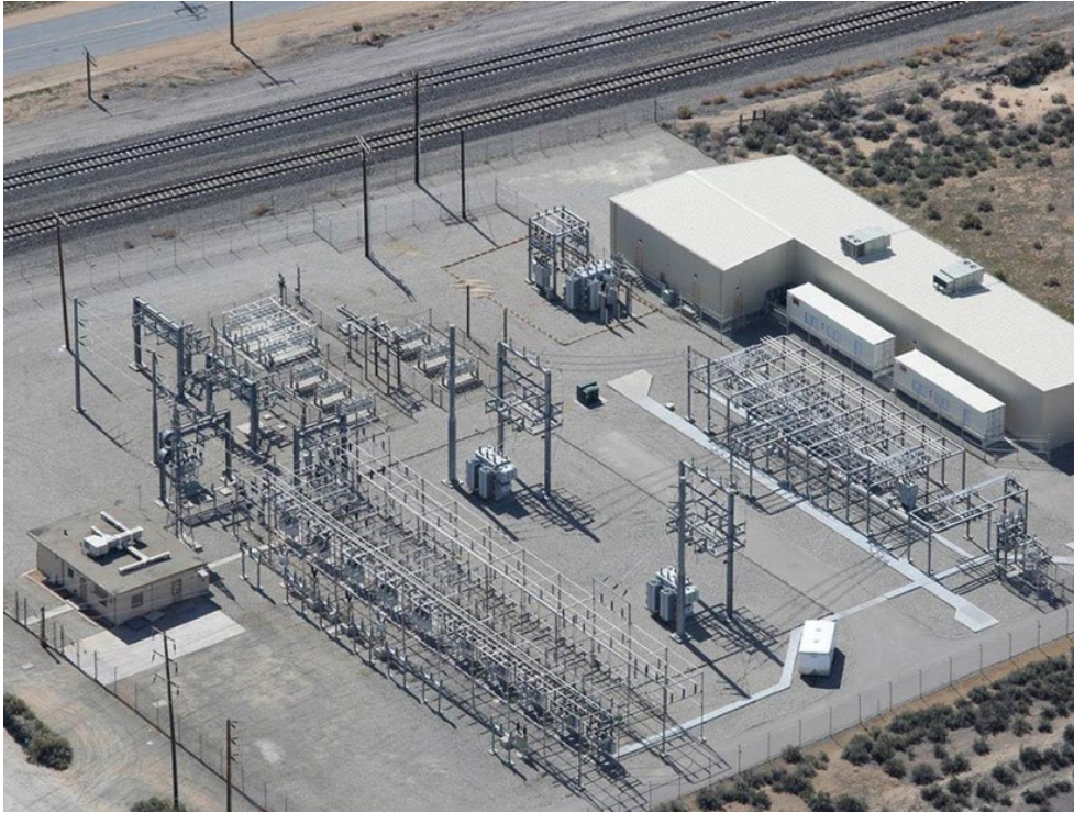
The Tehachapi Energy Storage Project is a lithium-ion battery energy storage system at the Monolith Substation of Southern California Edison in Tehachapi, Calif. | Sandia National Laboratories
