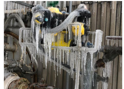
Frozen instrumentation at an Entergy power plant | Entergy
