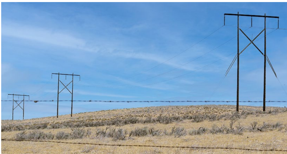
BPA transmission line in Umatilla County, Ore. | © RTO Insider LLC
