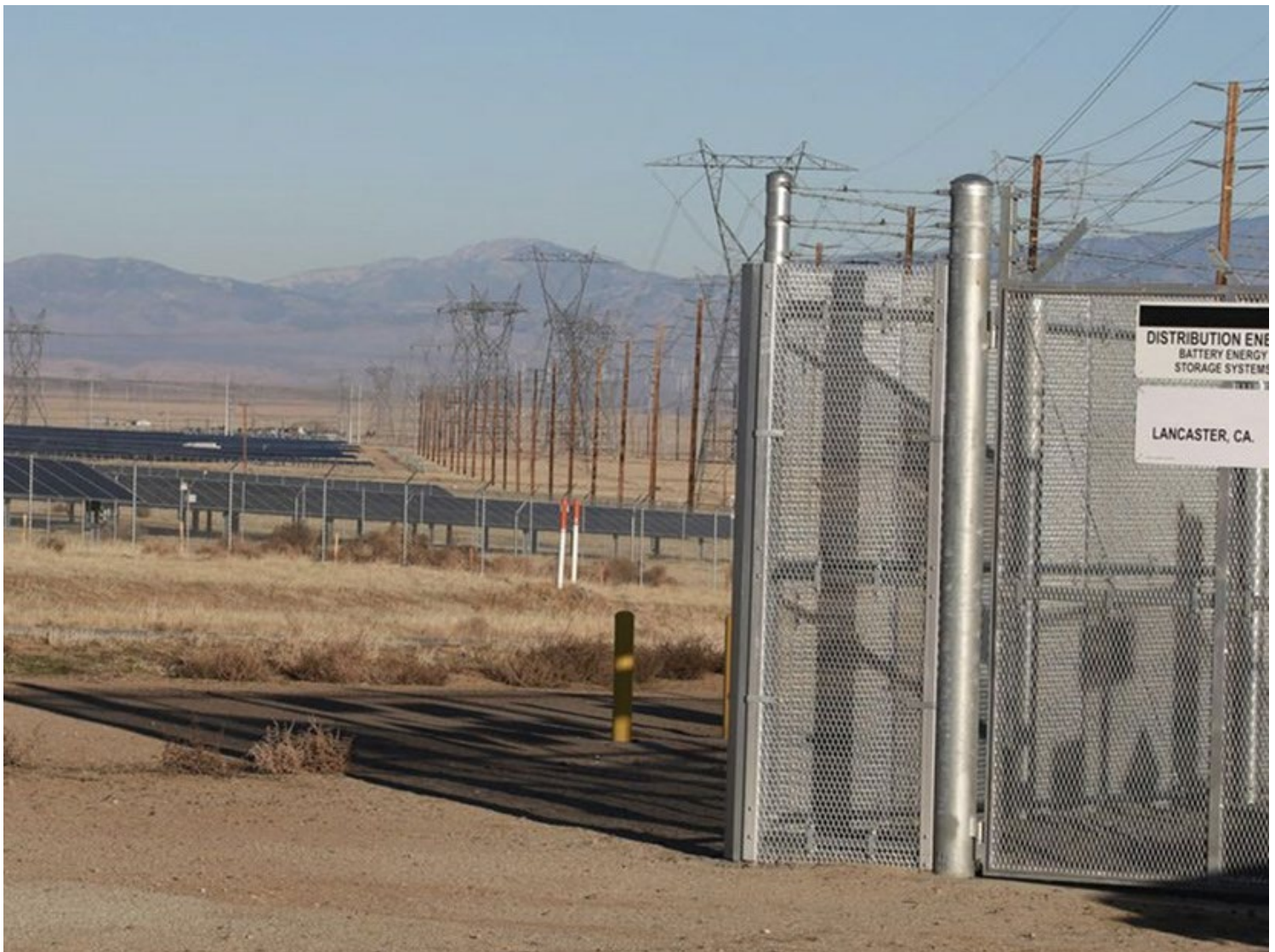
The Connolly Energy Storage System of Southern California Edison is located on the Pronghorn Circuit near 15 solar farms. | Southern California Edison
