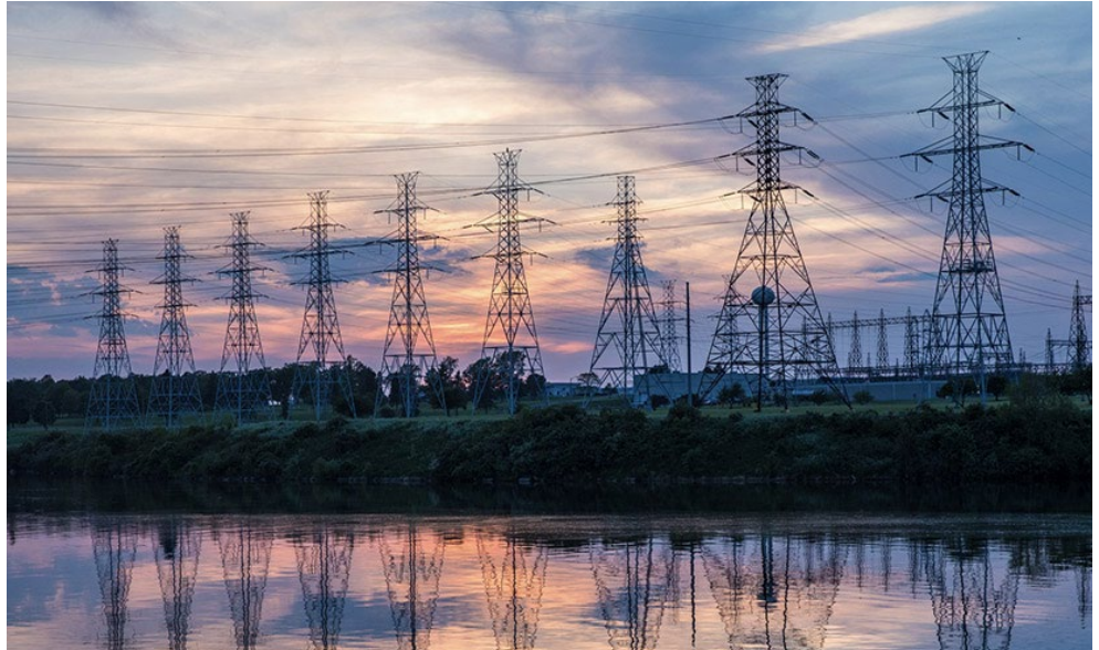
New York is investing hundreds of millions of dollars upgrading transmission lines like these to modernize the electric power grid. | NYPA
