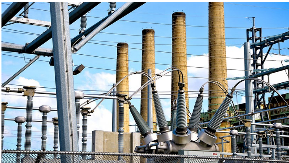
PSEG's Sewaren combined cycle plant in New Jersey. | PSEG
