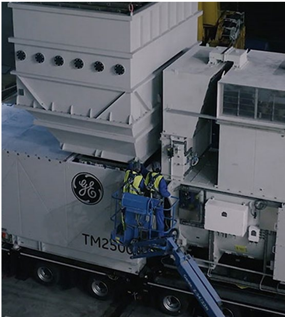
Part of the CPUC’s plan would allow PG&E to lease more mobile generating units. | General Electric
