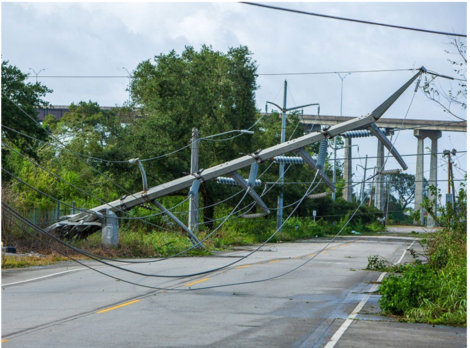
Hurricane Ida damage in New Orleans on Aug. 30 | Entergy
