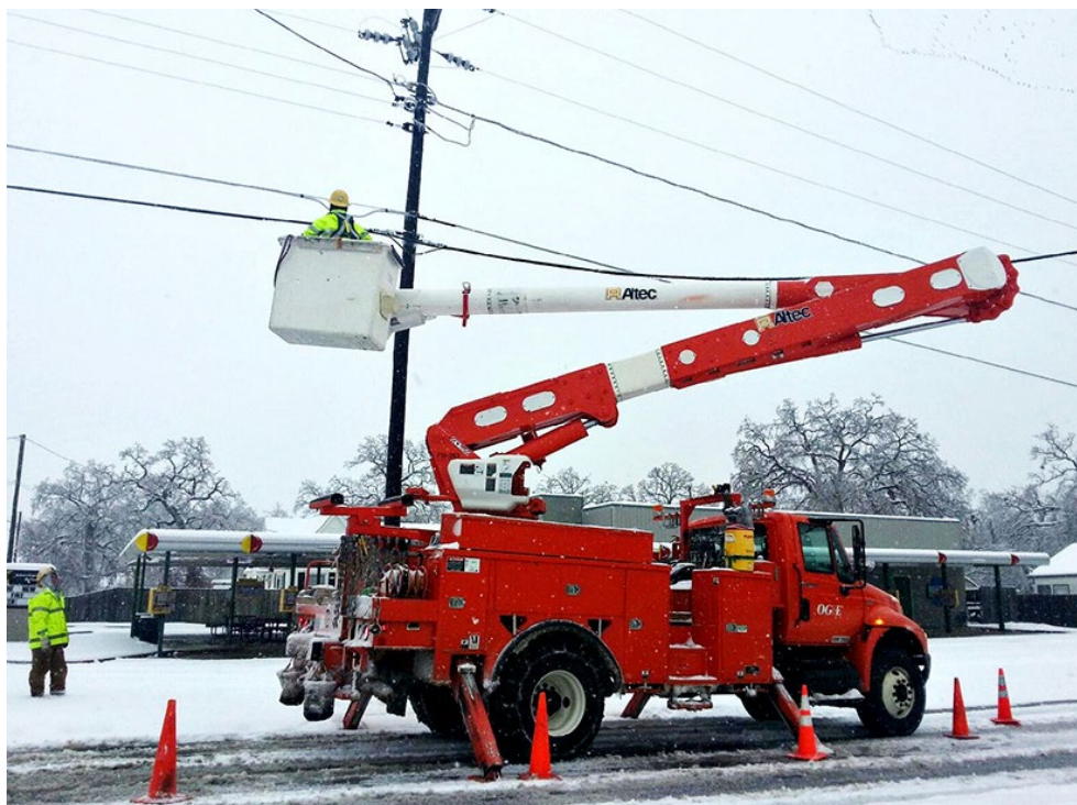
OG&E service crew works on restoring service following Winter Storm Uri. | OG&E
