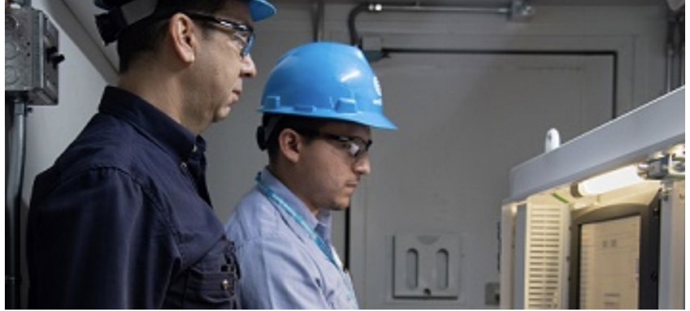
Con Edison senior engineers Steven Goldman (left) and Jorge Tua inside a company battery storage unit in Ozone Park, Queens. | Con Edison
