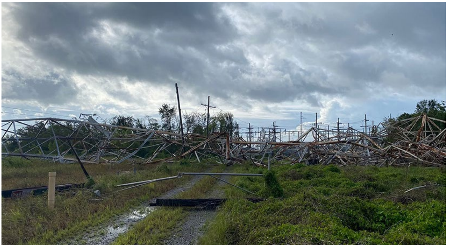
Damage from this year's Hurricane Ida in Louisiana | Entergy
