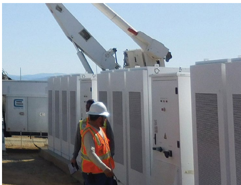
The CPUC's procurement order included increased battery storage | PG&E
