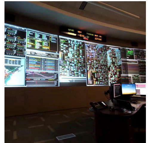
MISO control room | MISO
