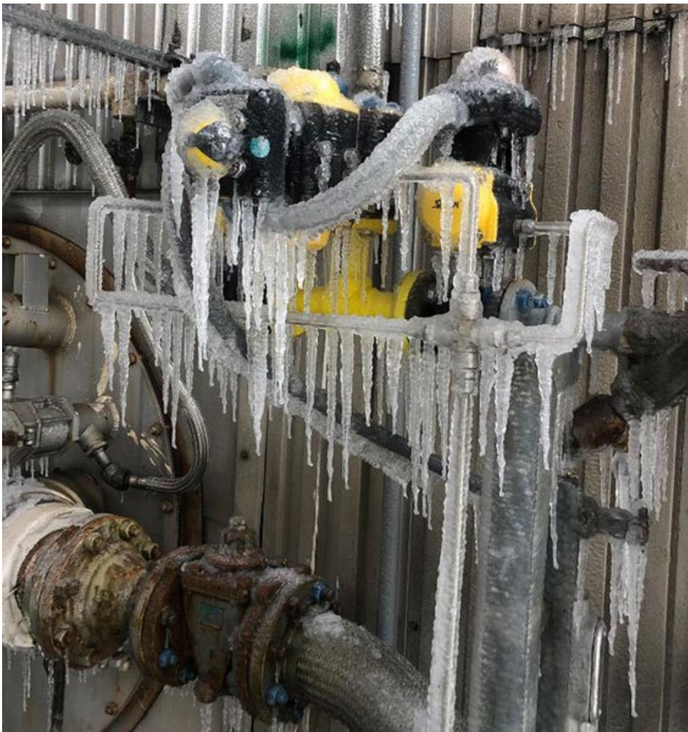
Frozen instrumentation on a Texas power plant during February's winter storm | Entergy
