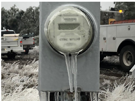
ERCOT's transmission operators have all filed their winter readiness reports. | Kerrville PUB
