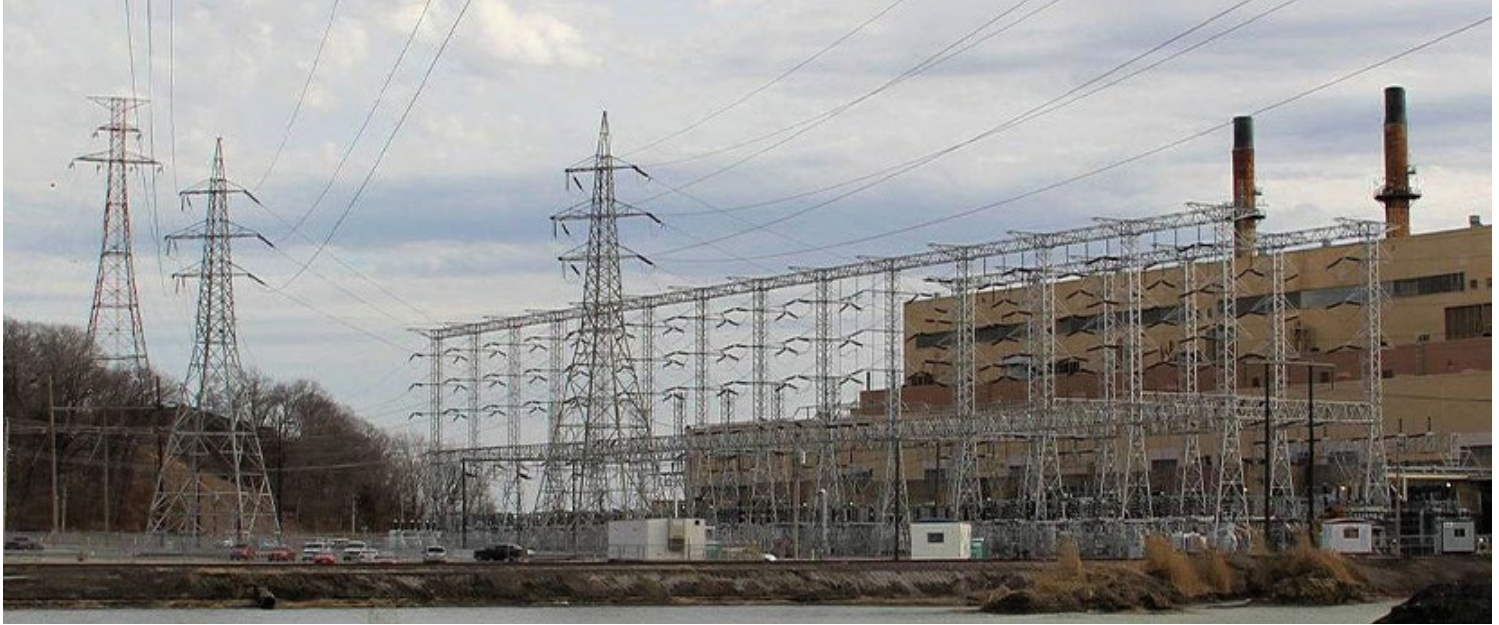
Ameren's coal- and gas-fired Meramec Power Plant | Missouri State Representative Jim Murphy
