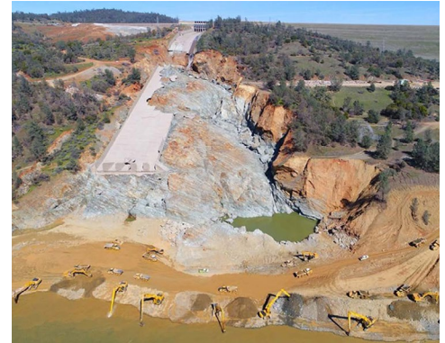
Ultimate damage at the Oroville service spillway | California Department of Water Resources
