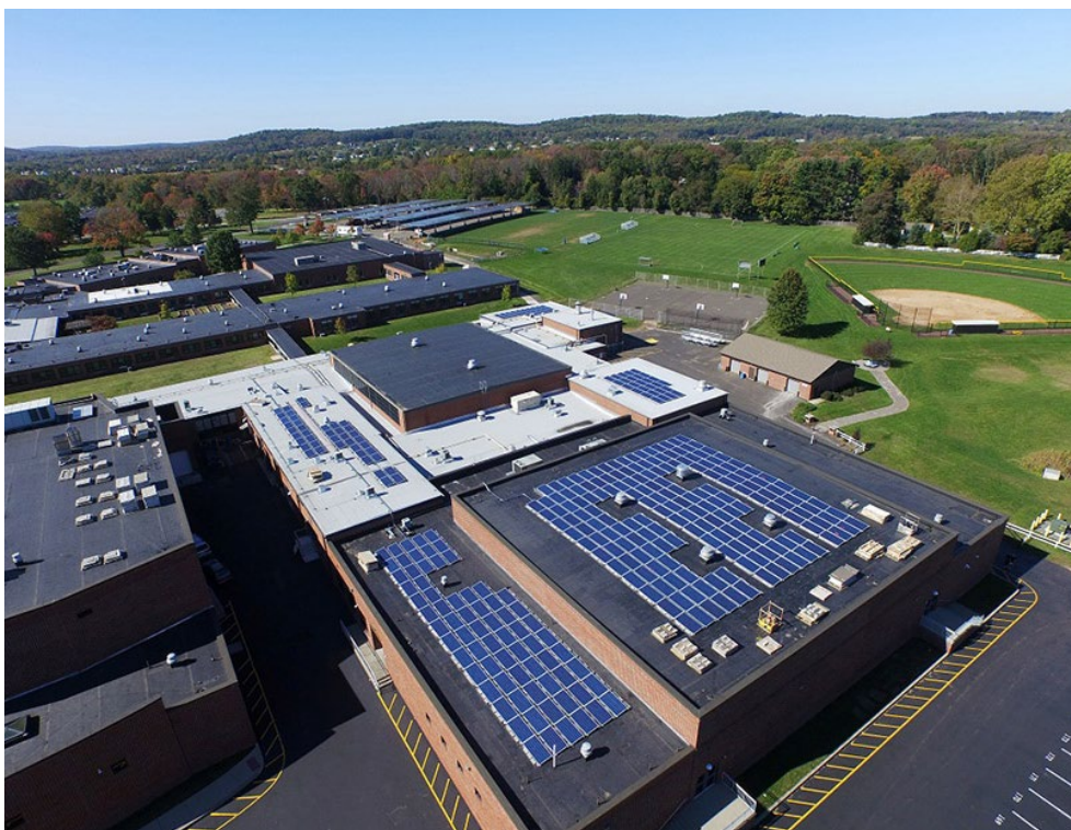
An 876-kW solar installation in Hopewell, N.J. | Advanced Solar Products
