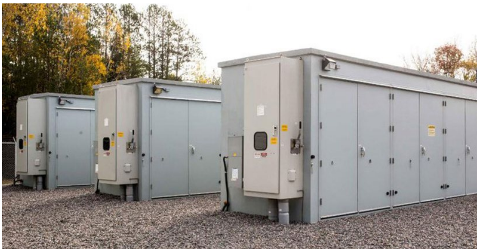
NextEra Energy is developing 2.4 GW of battery storage in California for deployment in 2023-2024. | NextEra Energy Resources
