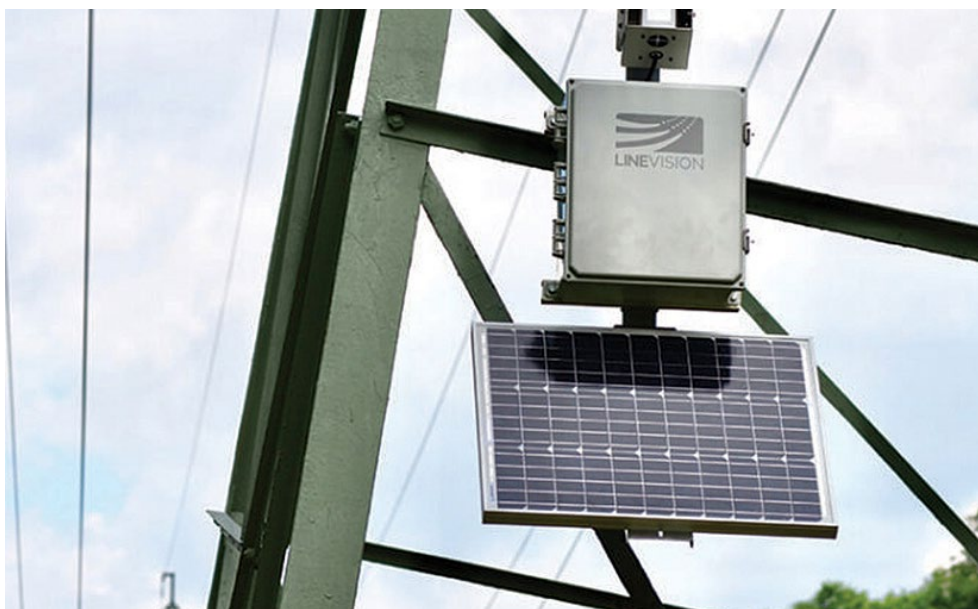
Dynamic line ratings, such as those provided by LineVision's overhead line monitoring system, can allow increased transmission capacity and provide grid operators with real-time situational awareness of potential problems. | LineVision
