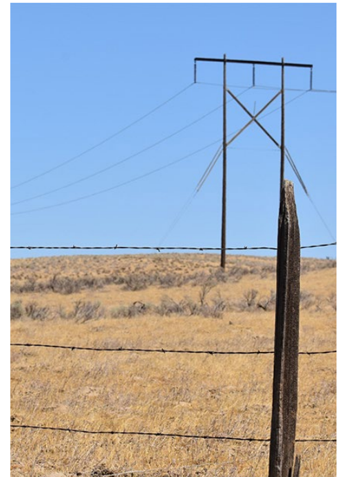
Transmission line in Umatilla County, Ore. | © RTO Insider LLC
