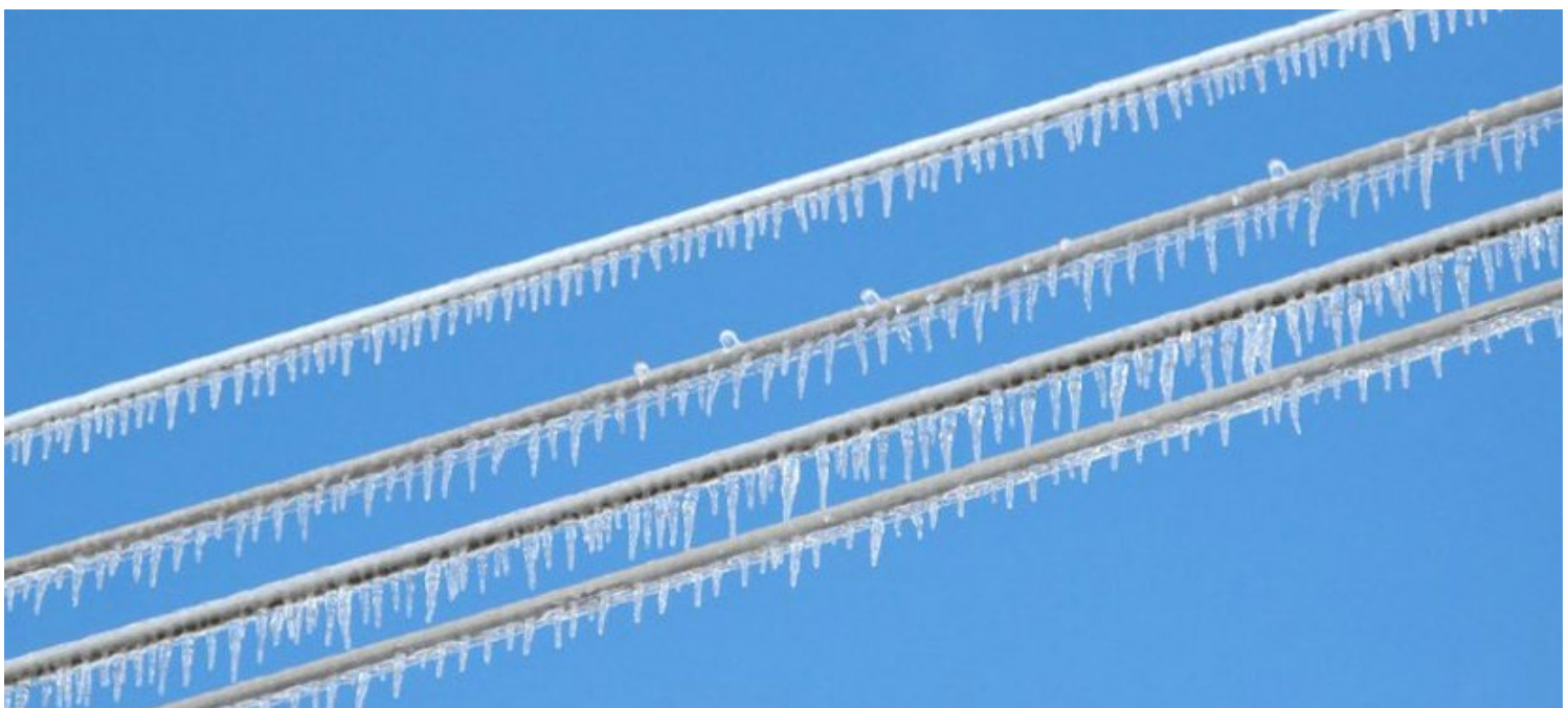
Frozen transmission lines after February's winter storm | Entergy
