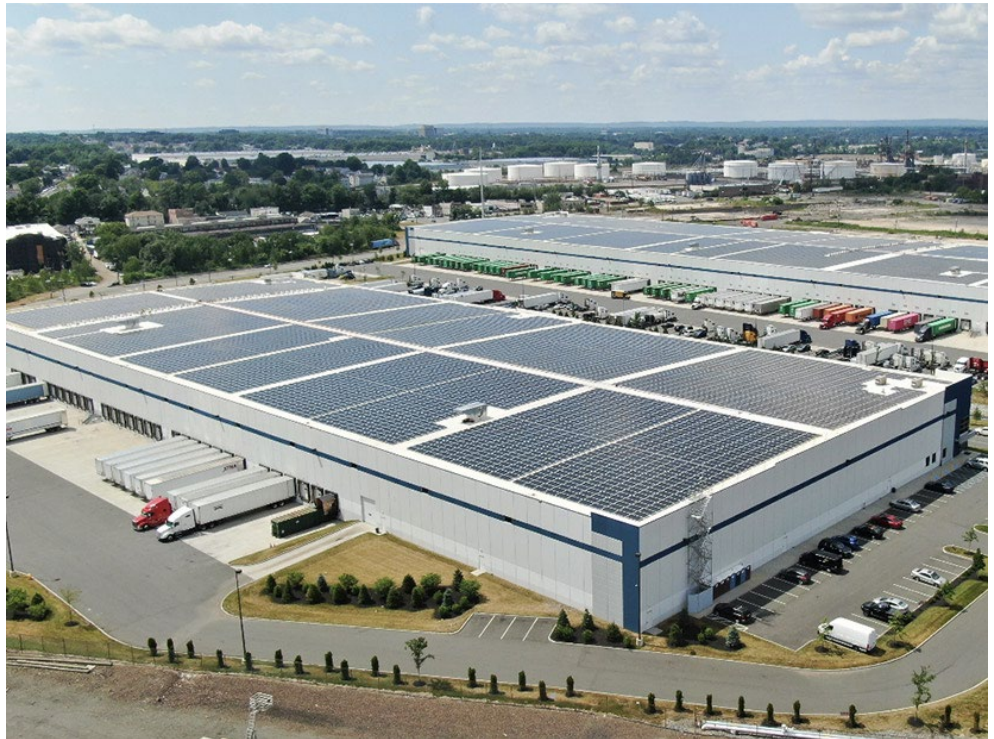
A solar project installed on a warehouse rooftop in Perth Amboy as part of New Jersey's Community Solar Energy Pilot Program | Solar Landscape
